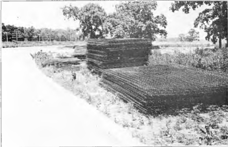
Fig. 2. Roadside stock pile of welded wire fabric. Illustrating convenient storage and handling of reinforcement when finished in flat, rigid sheets.
