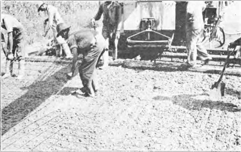
Fig. 4. Placing sheets of reinforcement. The flat sheets of reinforcement are being placed on the rough-struck bed of concrete.
