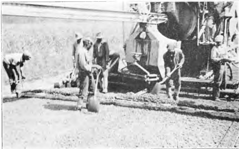
Fig. 3. Striking off concrete preliminary to installing sheet reinforcement. Concrete has been deposited on the subgrade and given a preliminary strike-off at an elevation 2 inches below final pavement surface.
