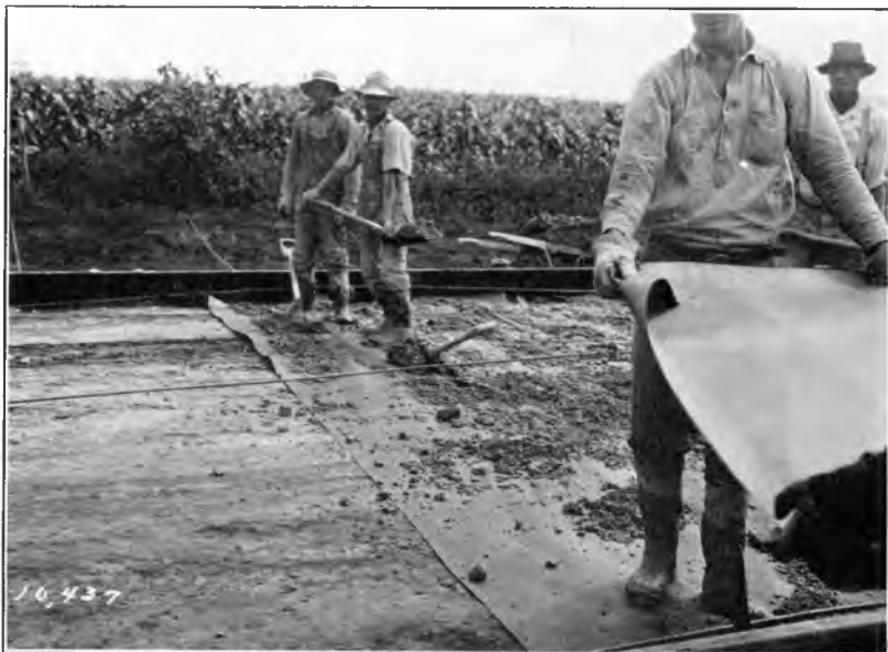
Fig. 4. Layer of tar paper specified on all subgrades for concrete road slabs.
