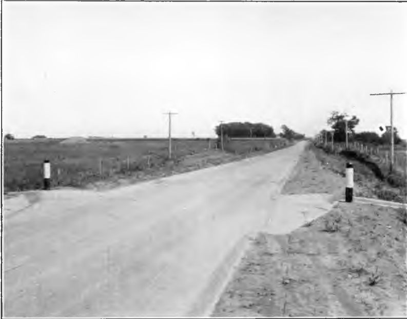
Fig. 2. Wide throated, flat section flume to direct water from pavement at sags in grade.
