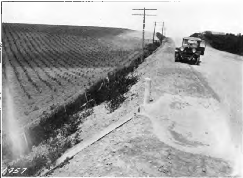
Fig. 3. Cars running on shoulder can pass over this flat section flume without damage.
