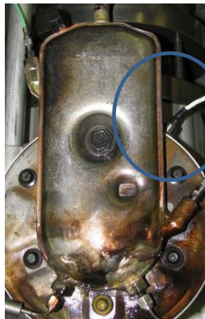
Figure 3. Pressure transducer mounted to suction plenum.
