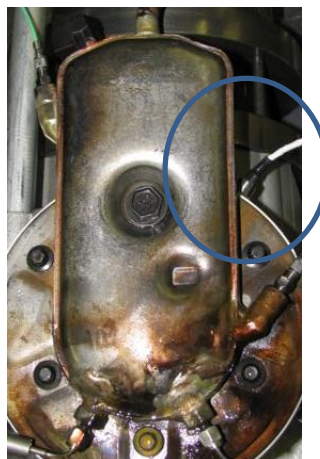
Figure 3. Pressure transducers mounted to suction plenum.
