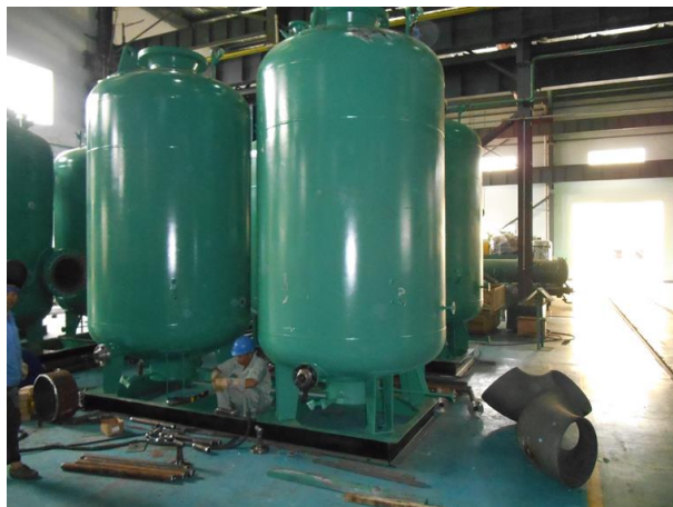
Figure 6: Oil Separator Skid
