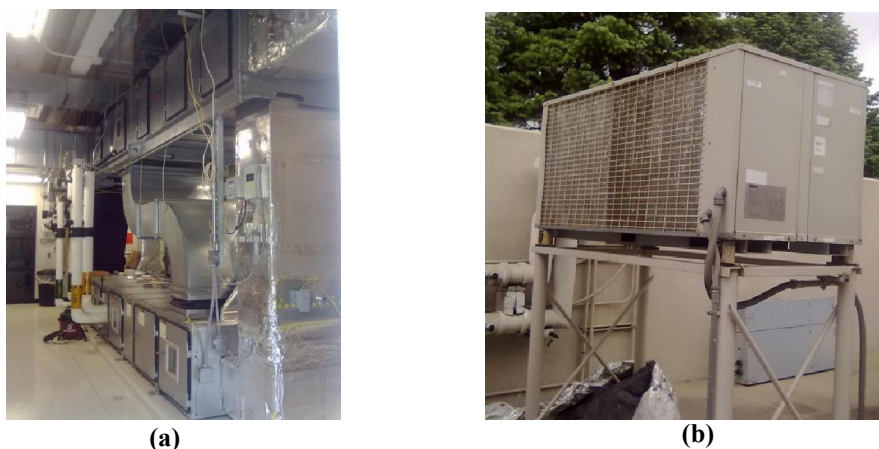
Figure 9: (a) Overview of air-handling unit (b) Overview of air-cooled liquid chiller
