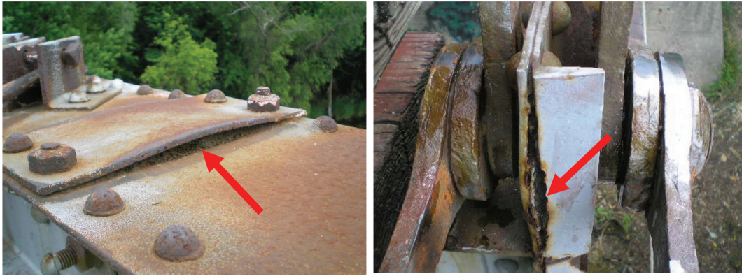
Figure 3.37 Pack rust in mechanically fastened connections.
