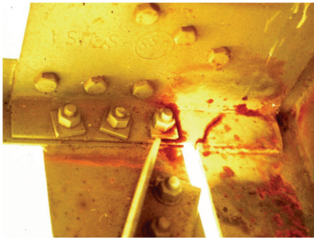
Figure 3.43 Cracking in flange of channel (gusset plate) and girder.
