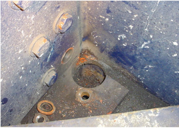
Figure 3.31 Retrofit hole (prior to finish grinding). (Note guide plate used as template to ensure core barrel does not “wobble”.)
