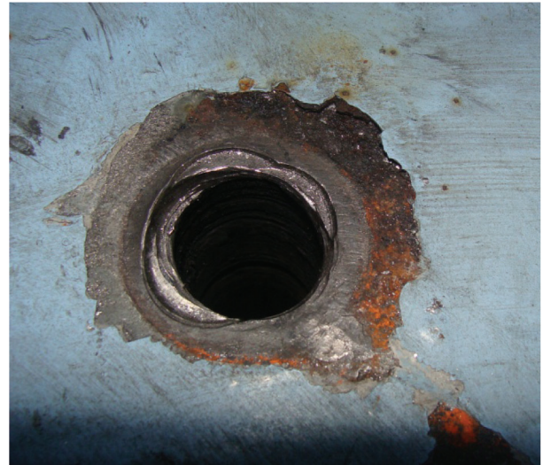
Figure 3.41 Damaged surface after rivet removal around hole (courtesy of Purdue University).
