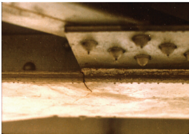
Figure 3.44 Cracking in girder flange.
