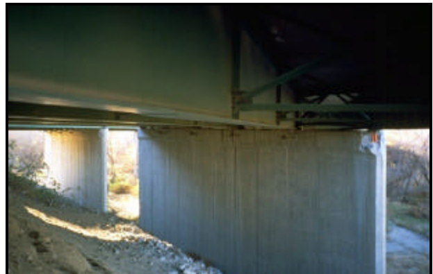
FIGURE 5.40 Spalling near location of anchor bolts after Northridge Earthquake 1994 (11)
