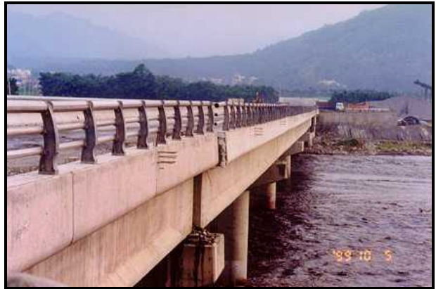
FIGURE 5.51 Transversal movement of bridge deck after Taiwan EQ (15)
