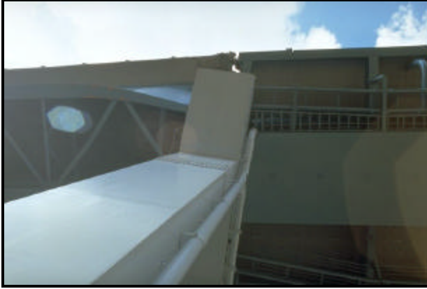
FIGURE 5.31 Buckling of steel girders (11)
