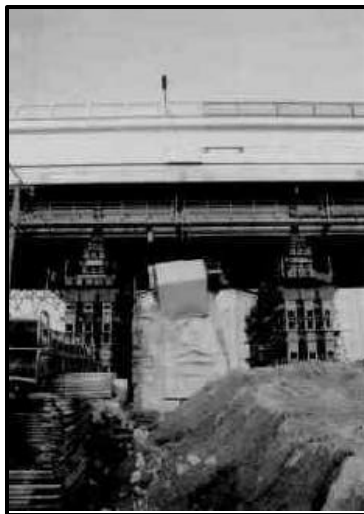
FIGURE 7.10 View of temporary shoring to prevent total collapse of bridge (27)
