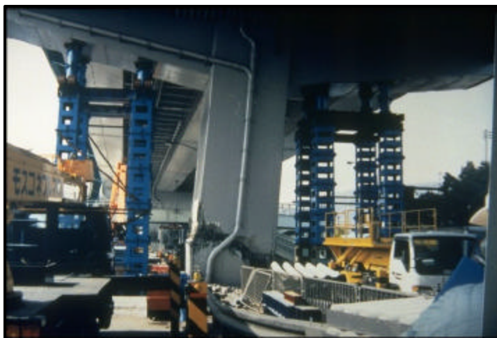
FIGURE 7.13 View of temporary support to prevent total collapse of steel girder bridge (11)
