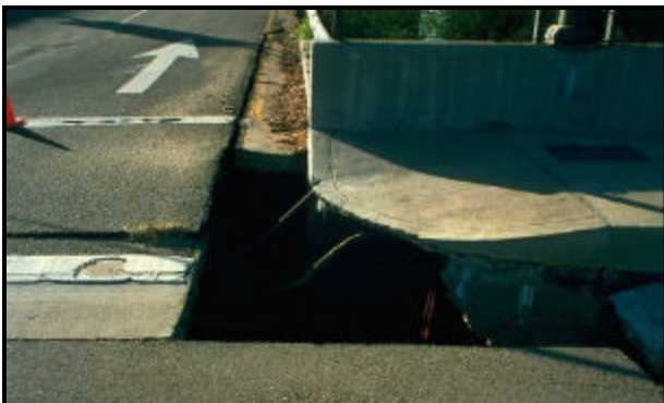
FIGURE 5.47 Collapse of asphalt pavement due to washout after Northridge EQ 1994 (11)
