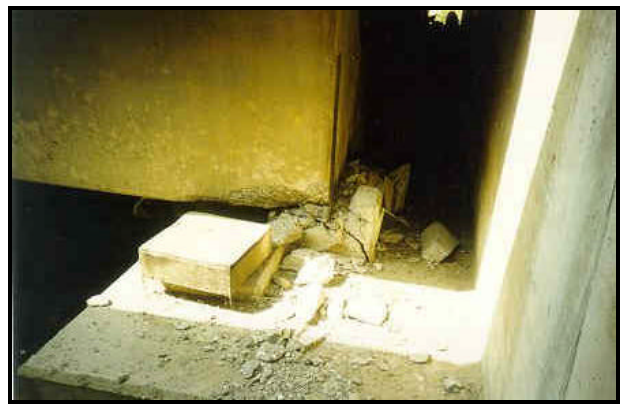
FIGURE 5.58 Sliding of elastomeric bearing (10)
