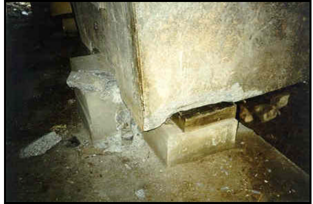
FIGURE 5.57 Elastomeric bearing movement and spalling of girder concrete (10)
