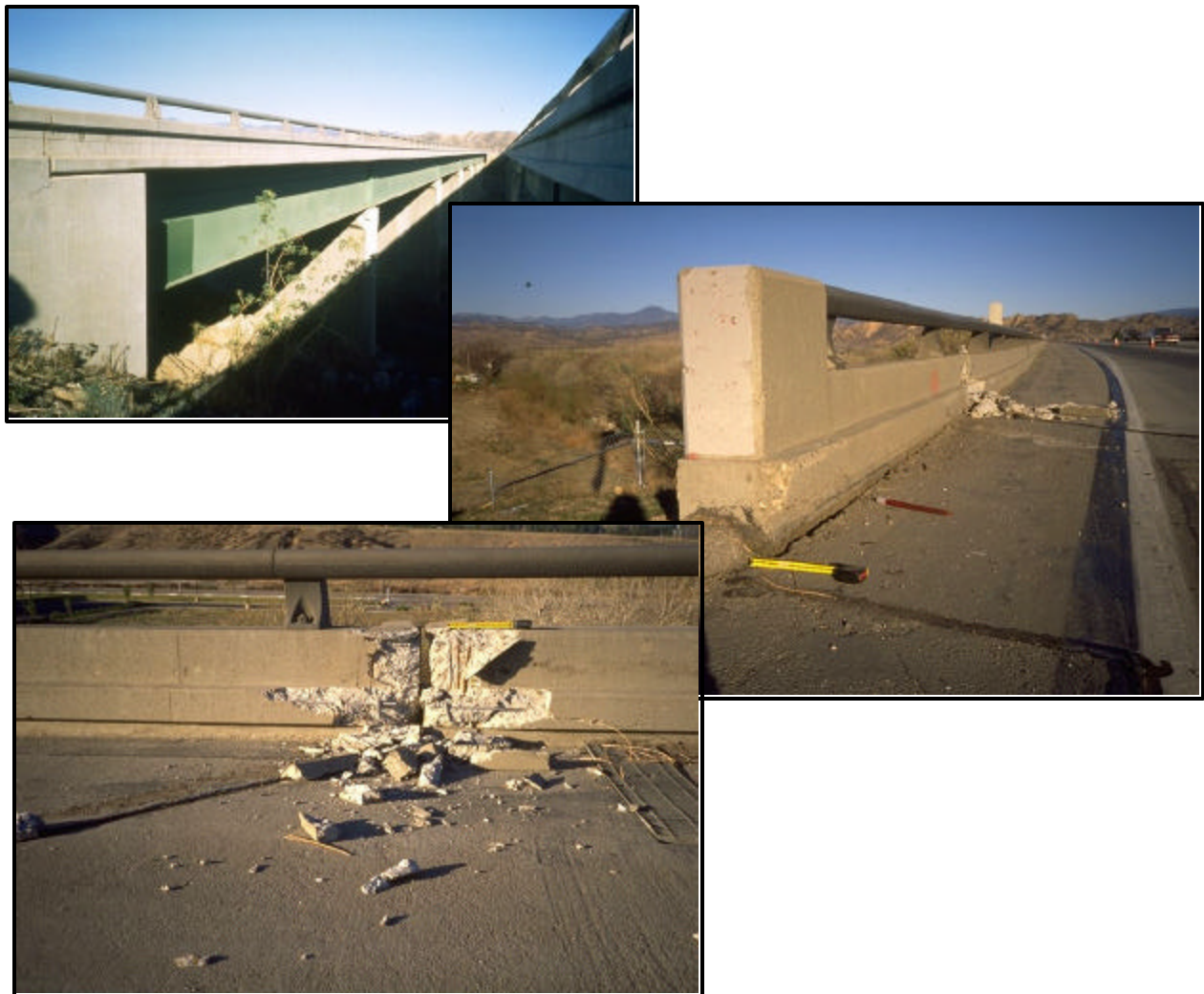
FIGURE 8.1 View of bridge superstructure after the earthquake (11)
