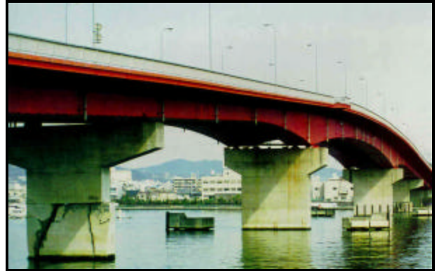
FIGURE 5.28 Heavy damage in RC bridge piers after Kobe Earthquake 1995 (14)
