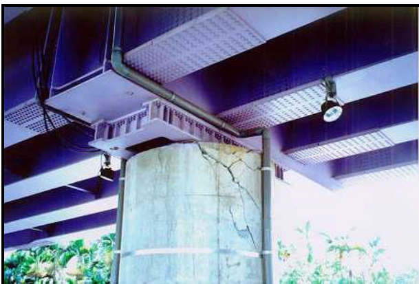
FIGURE 5.74 Compression failure on the top of RC bridge pier after Taiwan EQ 1999 (15)
