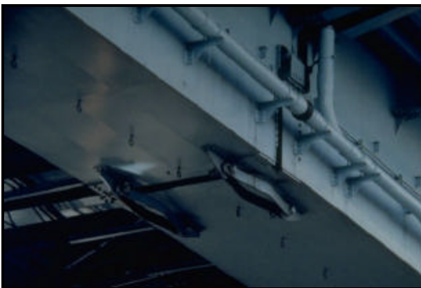
FIGURE 5.85 Buckled seismic restrainers (11)
