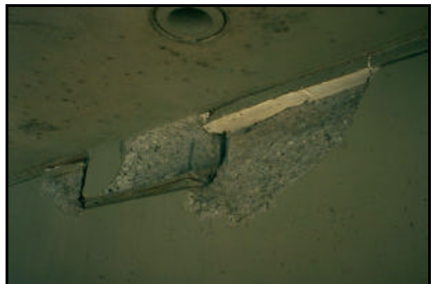
FIGURE 5.30. Shear key failure of a bridge piers after Northridge Earthquake 1994 (11)
