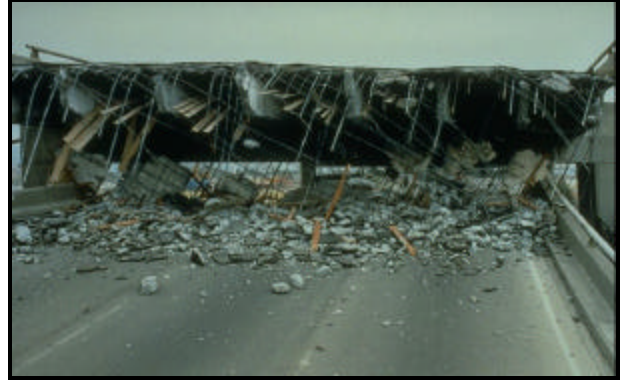
FIGURE 5.7. Failure of a monolithic RC girder bridge after Loma Prieta EQ 1989 (11)
