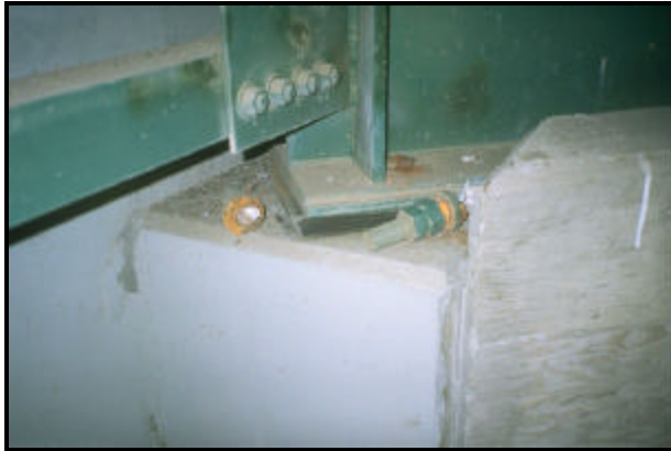
FIGURE 5.36 Failure of two anchor bolts for a girder after Northridge EQ 1994 (11)
