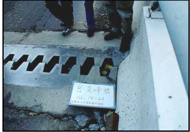
FIGURE 5.19 The expansion of the joints Taiwan EQ 1999 (15)
