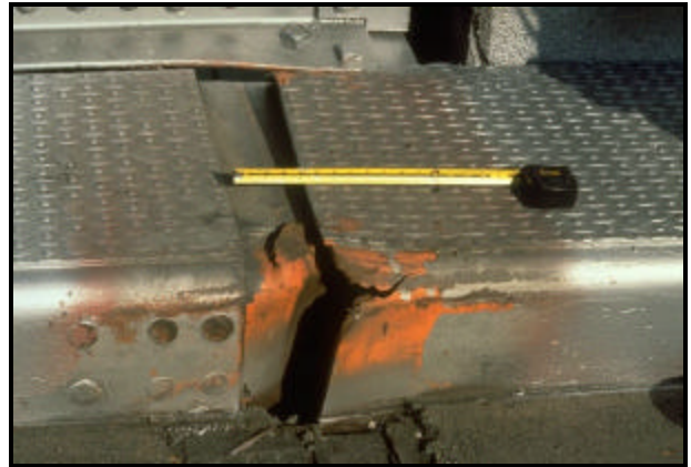
FIGURE 5.20 The expansion of the joints after Loma Prieta Earthquake 1989 (11)
