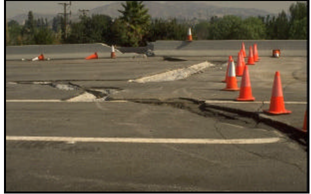
FIGURE 5.48 Surface damage to highway pavement after Northridge EQ 1994 (11)
