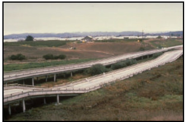
FIGURE 5.8 Collapse of RC girder bridge after Loma Prieta EQ 1989 (11)
