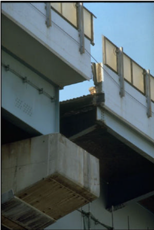
FIGURE 5.13 Excessive longitudinal movement of steel box girder bridge (11)
