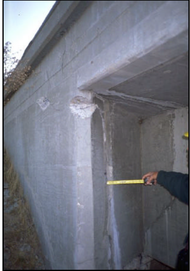
FIGURE 5.75 Separation of the superstructure and the abutment (11)
