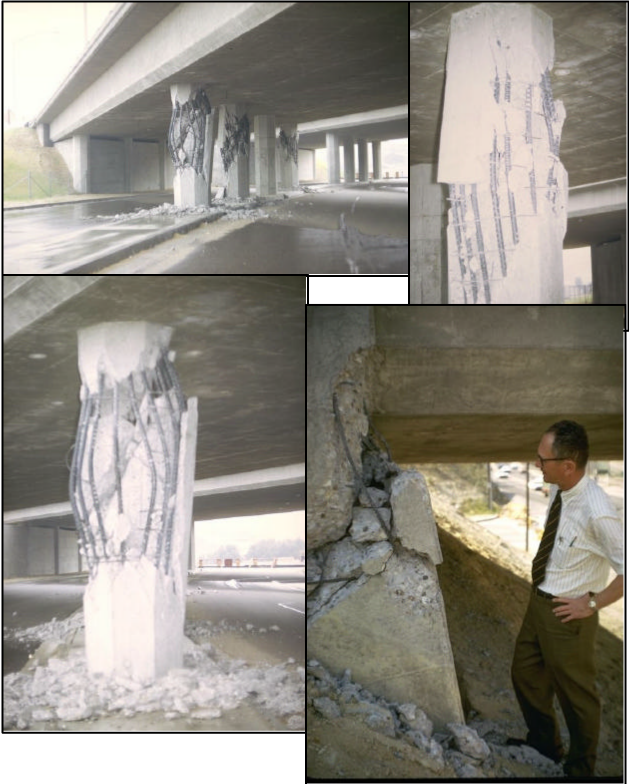
FIGURE 8.15 Substructure damage of the bridge (11)
