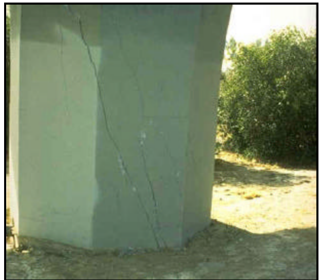
FIGURE 5.29 Shear crack in bents after Northridge Earthquake 1994 (11)
