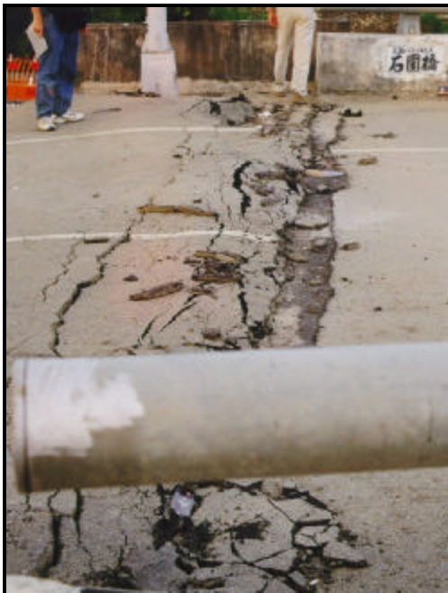
FIGURE 5.50 The cracking of pavement due to pounding and settlement the bridge (15)
