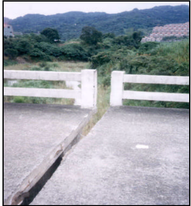
FIGURE 5.11 Excessive longitudinal movement of the bridge deck (15)
