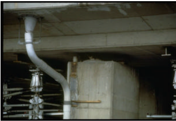
FIGURE 5.55 Shift of bearings after collapse (11)
