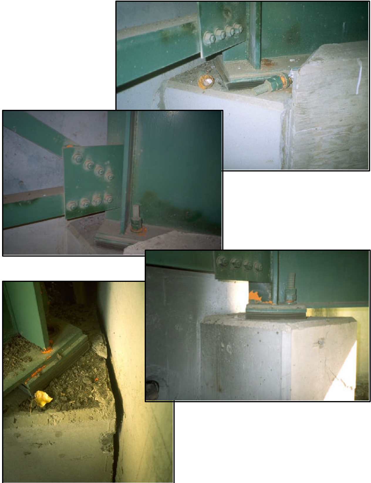
FIGURE 8.7 Damage to the bridge bearings (11)
