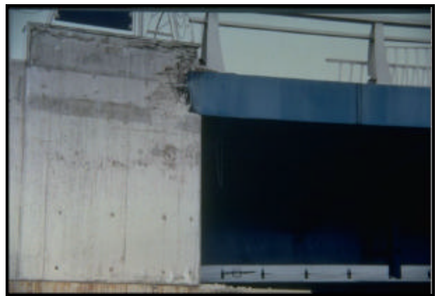
FIGURE 5.35 Pounding damage at abutment (11)
