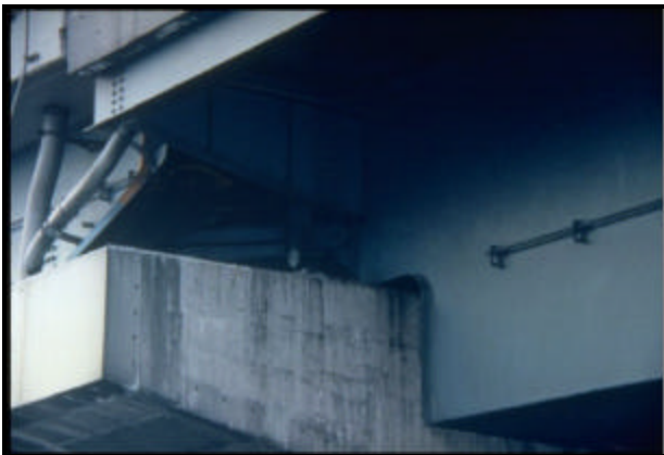
FIGURE 5.64 Steel box girder movement and collapse of bearings (11)
