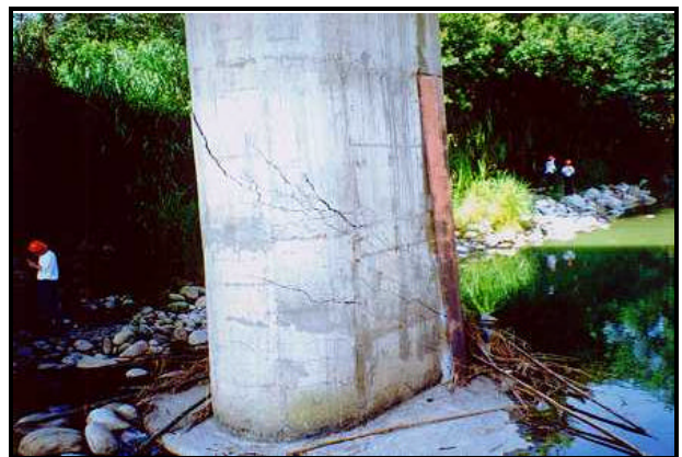
FIGURE 5.76 Heavily damaged RC bridge pier (15)
