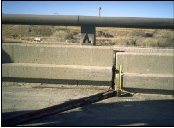
FIGURE 5.17 Vertical offset between decks after Northridge EQ 1994 (11)
