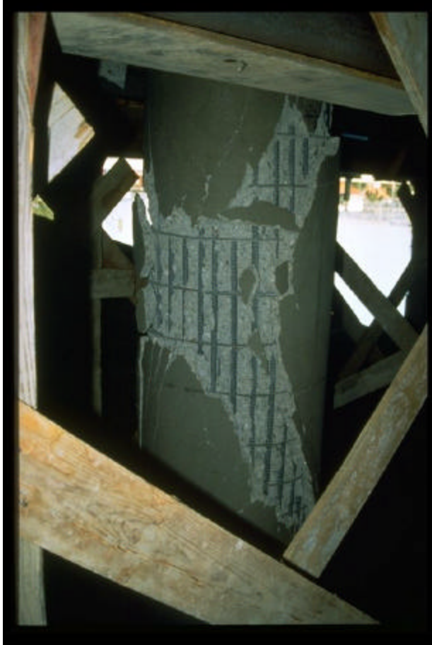
FIGURE 5.26 Failed RC bridge column (11)
