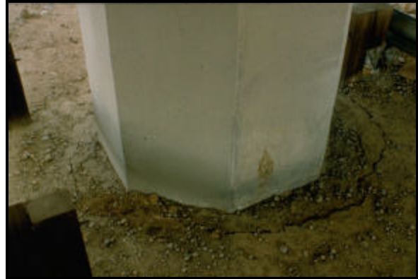
FIGURE 5.43 Disturbed soil at the base of column after Northridge EQ 1994 (11)
