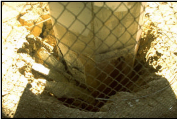
FIGURE 5.41 Separation of soil at column base of a pier after Northridge EQ 1994 (11)
