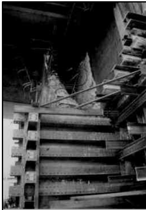
FIGURE 7.6 View of temporary shoring to prevent total collapse of bridge (27)
