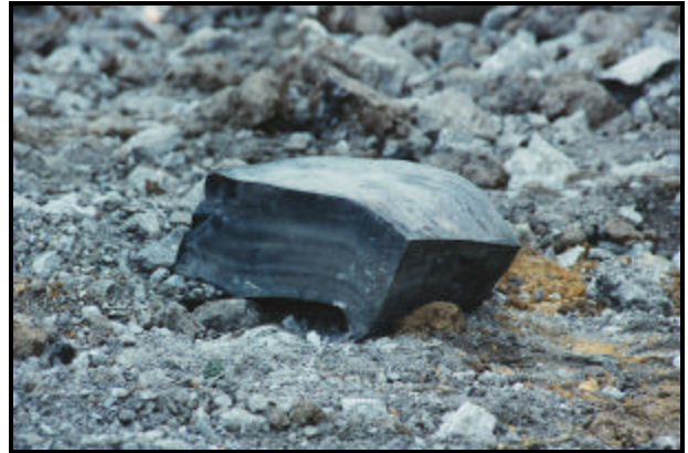
FIGURE 5.39 View of a failed elastomeric bearing pad after Izmit EQ 1999 (10)
