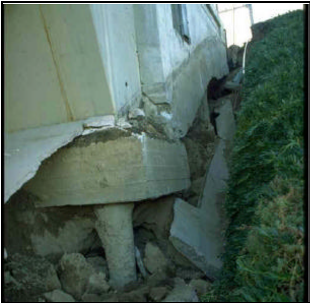
FIGURE 5.32 Movement of an abutment after Northridge Earthquake 1994 (11)
