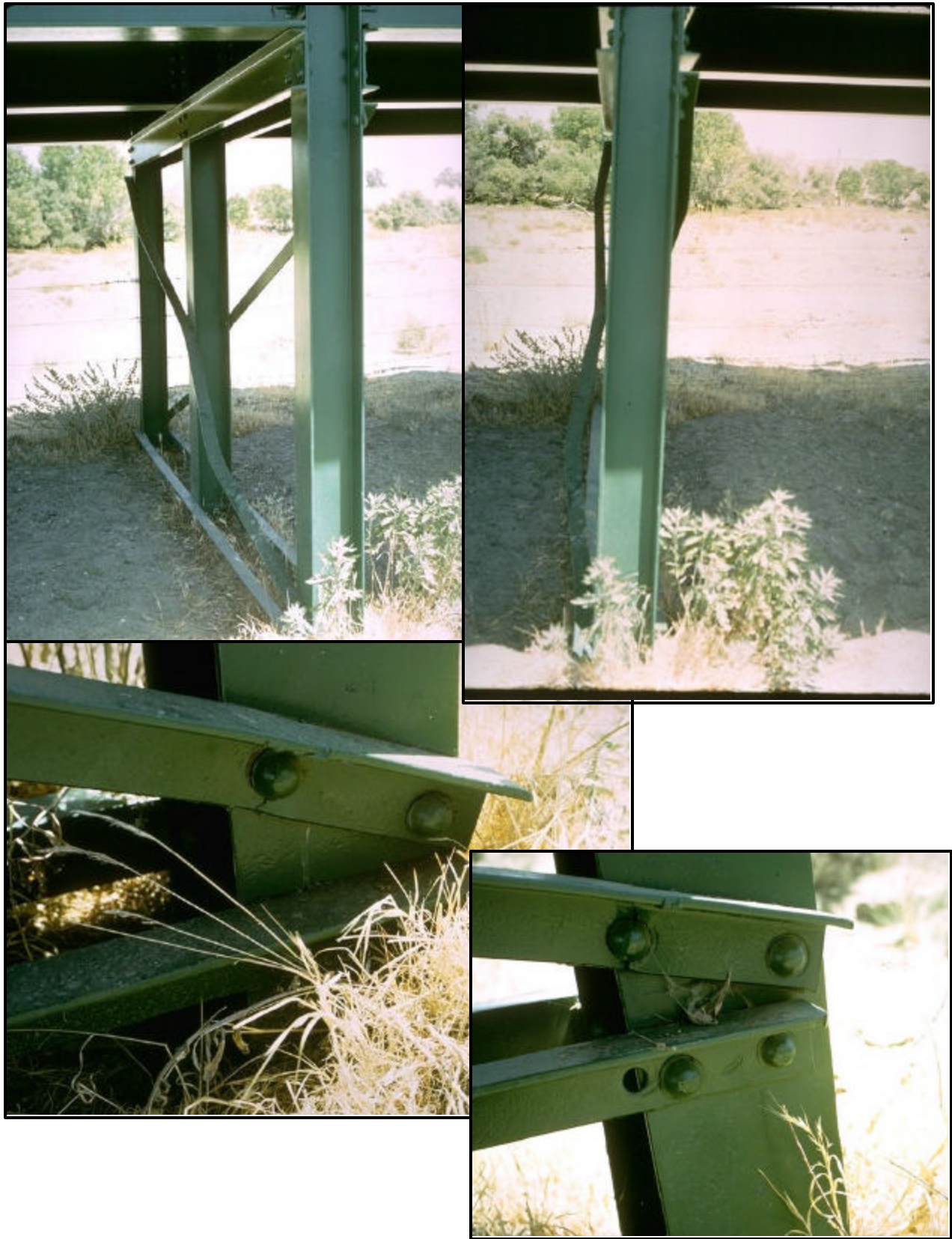
FIGURE 8.12 View of the damaged bridge components (11)
