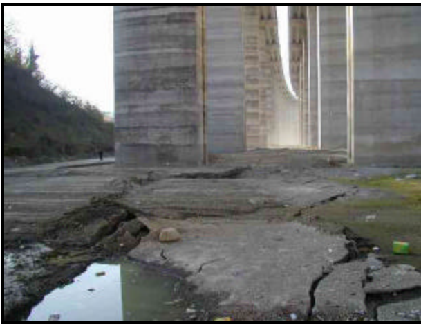
FIGURE 5.84 Soil failure due to the fault movement through RC bridge piers after Duzce EQ 1999 (10)
