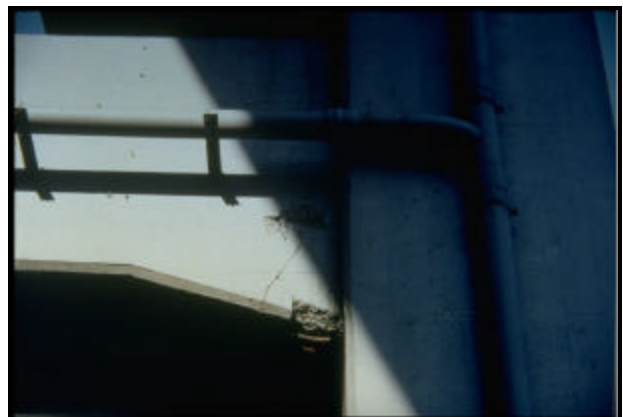
FIGURE 5.62 Damage at the bottom of the RC collector beam (11)
