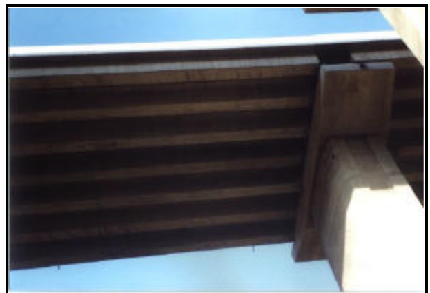
FIGURE 5.16 Longitudinal movement of RC box girders after Duzce EQ 1999 (10)
