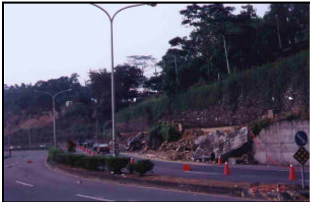
FIGURE 5.78 Retaining wall failure after Taiwan EQ 1999 (26)
