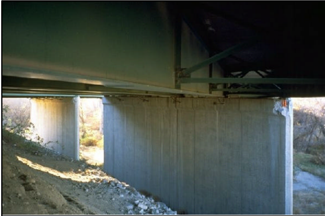
FIGURE 8.5 Damage to one of the bridge piers (11)
