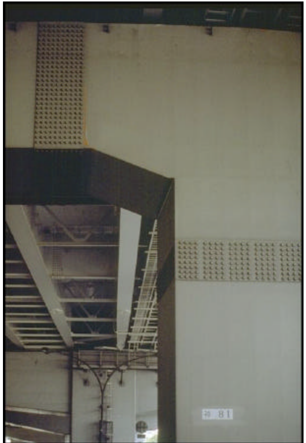
FIGURE 5.66 Yielding at bolted connector beam (11)
