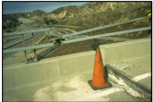
FIGURE 5.21 Vertical and horizontal offset on a bridge after Northridge EQ. 1994 (11)
