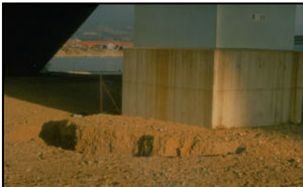
FIGURE 5.79 Settlement around RC bridge pier (11)
