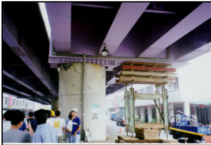
FIGURE 7.12 View of temporary support to prevent total collapse of steel girder bridge (15)
