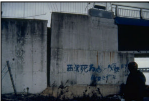
FIGURE 5.33 Separation of abutment (11)
