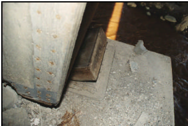
FIGURE 5.37 Failure of an elastomeric bearing due to longitudinal movement of girder (10)
