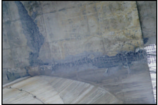
FIGURE 5.65 Heavy damage in RC box girder bridge (15)
