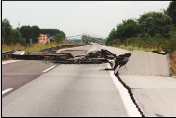
FIGURE 5.4 Collapse of roadway due to fault rupture after Izmit EQ 1999 (10)
