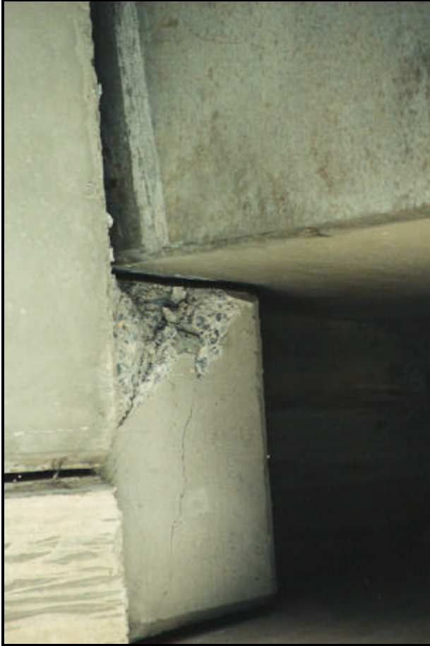
FIGURE 5.73 Concrete spalling and cracking due to pounding of RC box girder after Izmit EQ 1999 (10)
