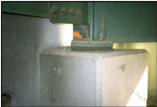
FIGURE 5.60 Buckling of web near lower flange and crack in pedestal (11)
