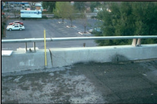
FIGURE 5.46 Curb separation after Northridge Earthquake 1994 (11)
