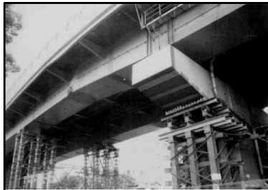
FIGURE 7.7 View of temporary shoring to prevent total collapse of steel bridge (27)
