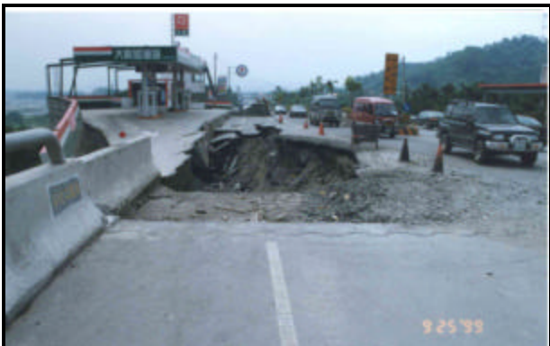
FIGURE 5.69 Abutment slumping after Taiwan EQ 1999 (26)
