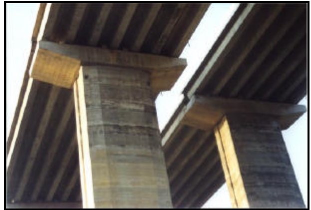
FIGURE 5.15 Lateral movement of prestressed RC box girders (10)
