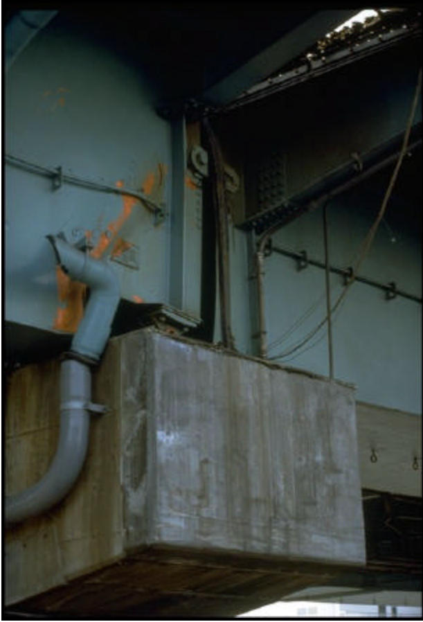
FIGURE 5.63 Buckling in the girder due to pounding (11)
