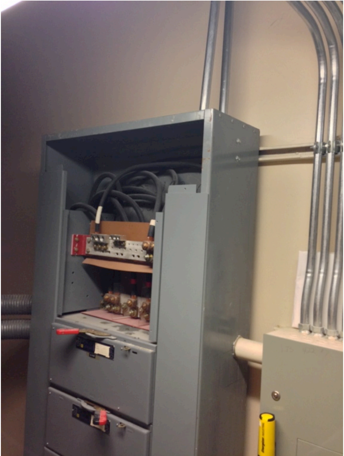
Figure C.16 Electrical Panel in Utility Room on Fourth Floor of Knoy Hall
