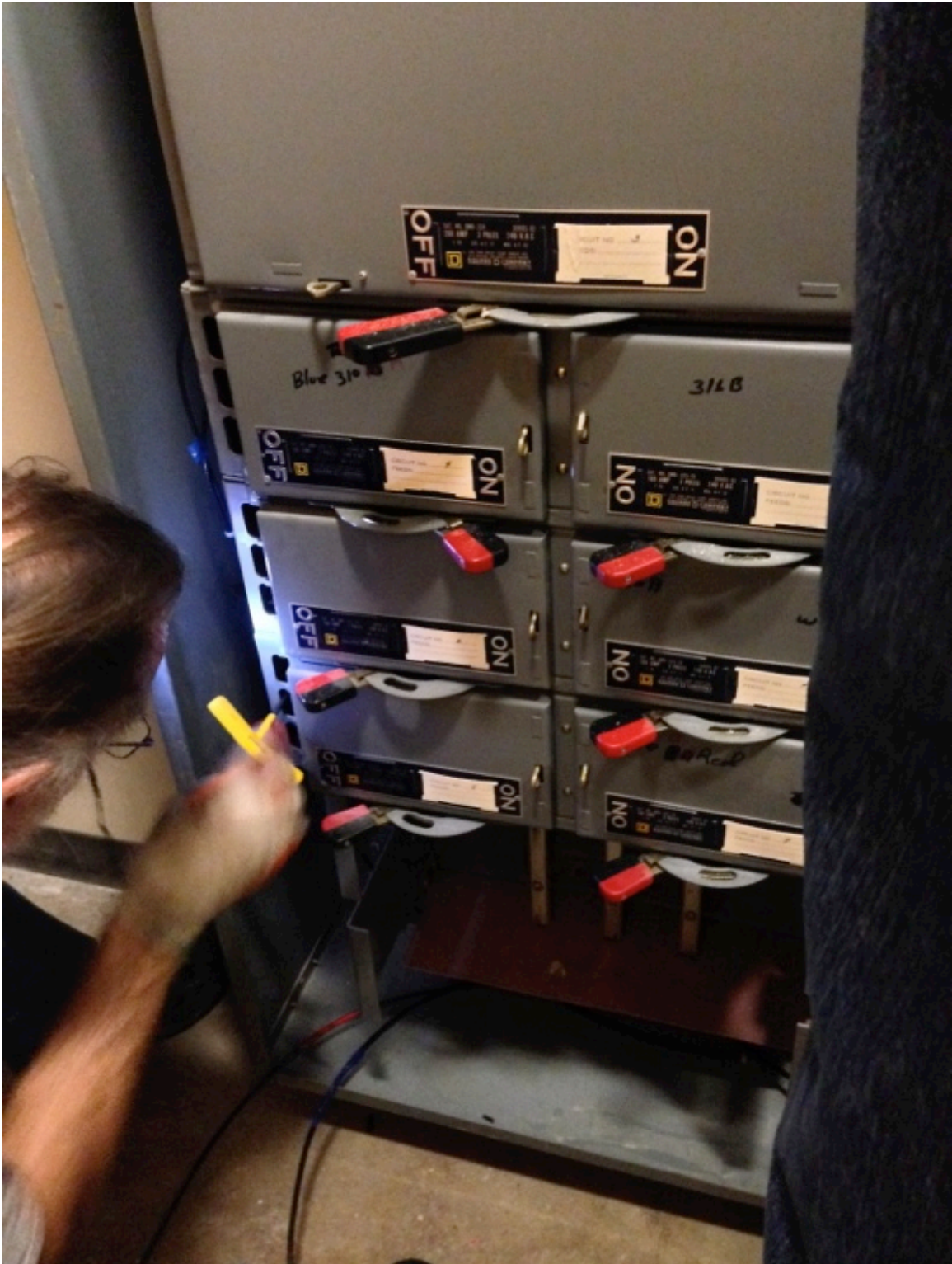
Figure C.17 Interconnection into the Electrical Panel
