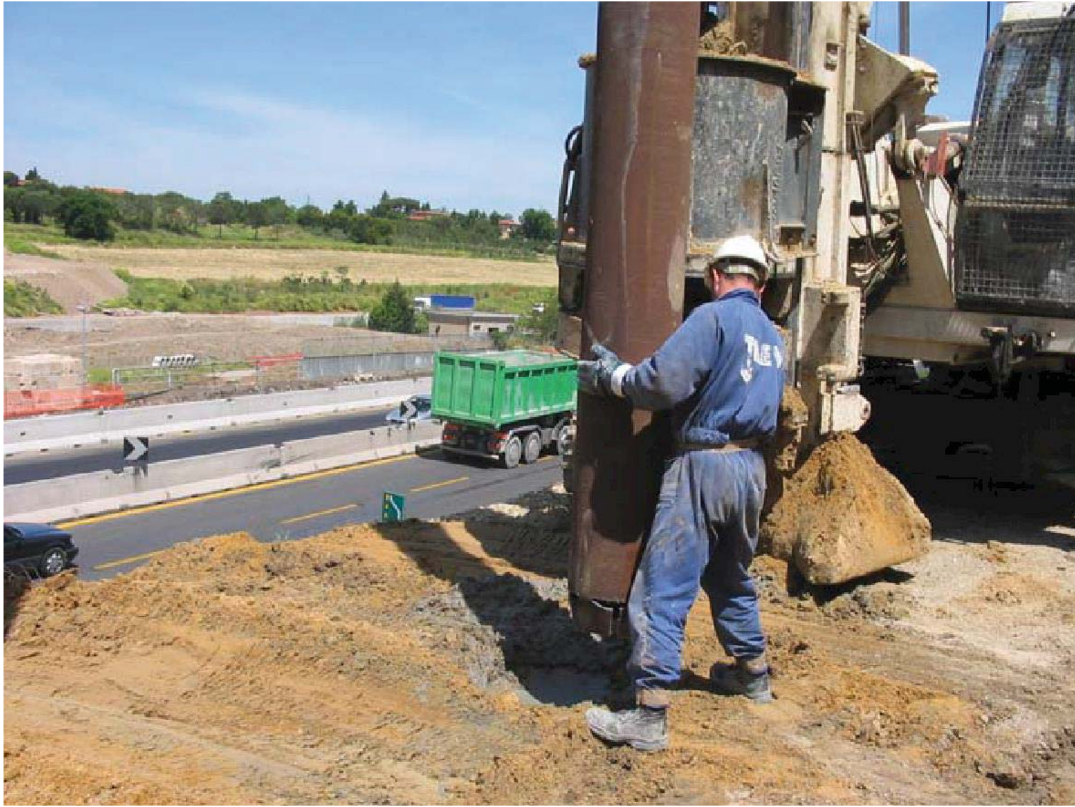
Use of Steel Pipe to Reinforce a CFA Pile for a Wall
