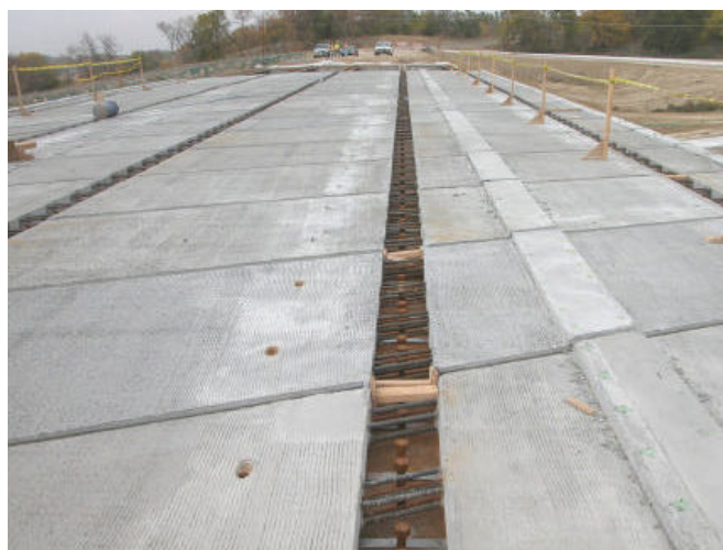
Figure 17 Open channel over girders for longitudinal post-tensioning on the Skyline Drive Bridge, Omaha, NE.
