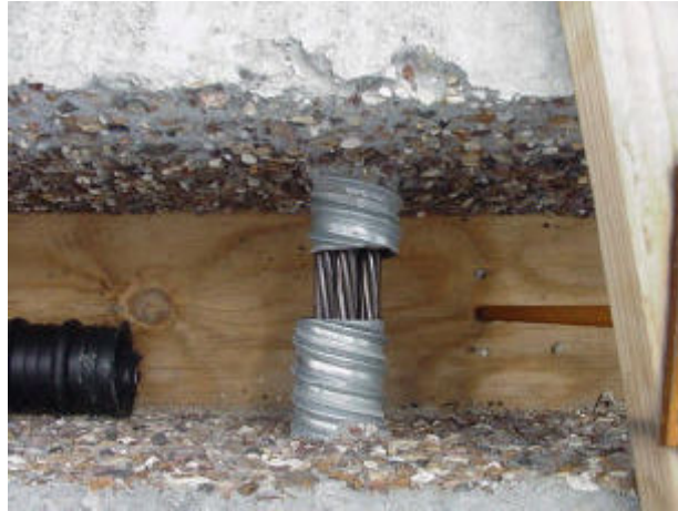
Figure 11 Exposed aggregate roughened surface.
