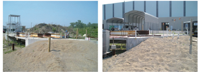
Figure B.8 Photos of the backfill behind the abutments.
