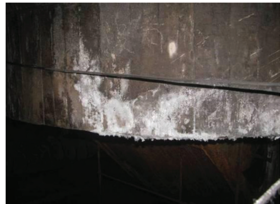
Figure 3. Funnel concrete surface with corrosive medium.
