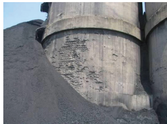
Figure 4. Damaged concrete wall of the bowl.
