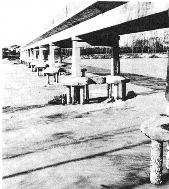
Figure 2.7 Degradation leads to bridge failure (after Galay, 1983)
