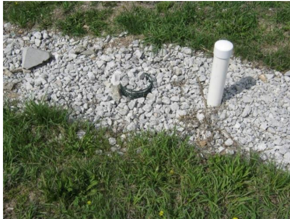
Figure 3.8 Upstream infiltration trench basket rock and observation well
