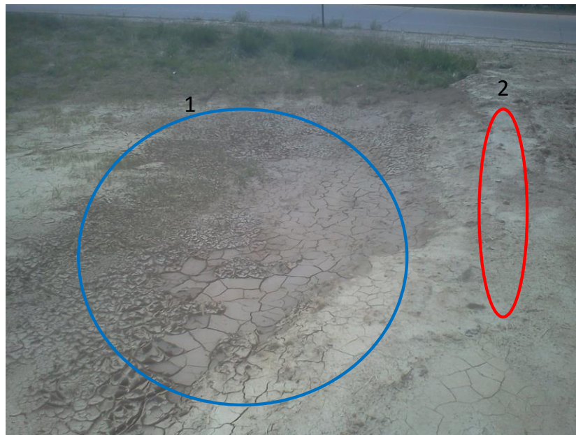
Figure 2.17 Check dam filter clogging
