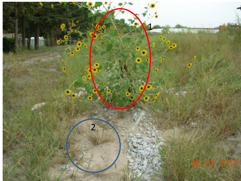
Figure 2.22 Filter trench sediment buildup and vegetative growth
