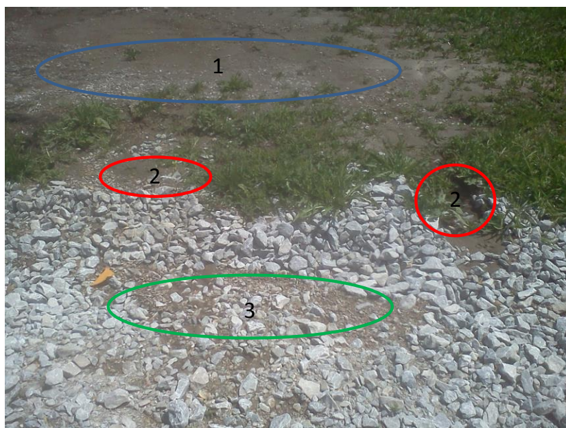
Figure 2.19 Infiltration trench clogging
