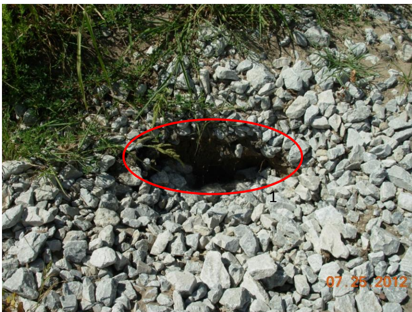
Figure 2.25 Filter trench undermining hole along trench
