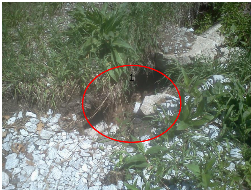
Figure 2.23 Filter trench undermining at beginning of trench
