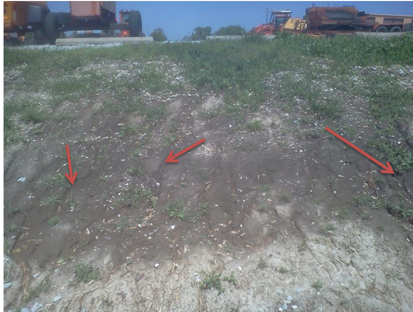
Figure 2.20 Filter trench side slope rills
