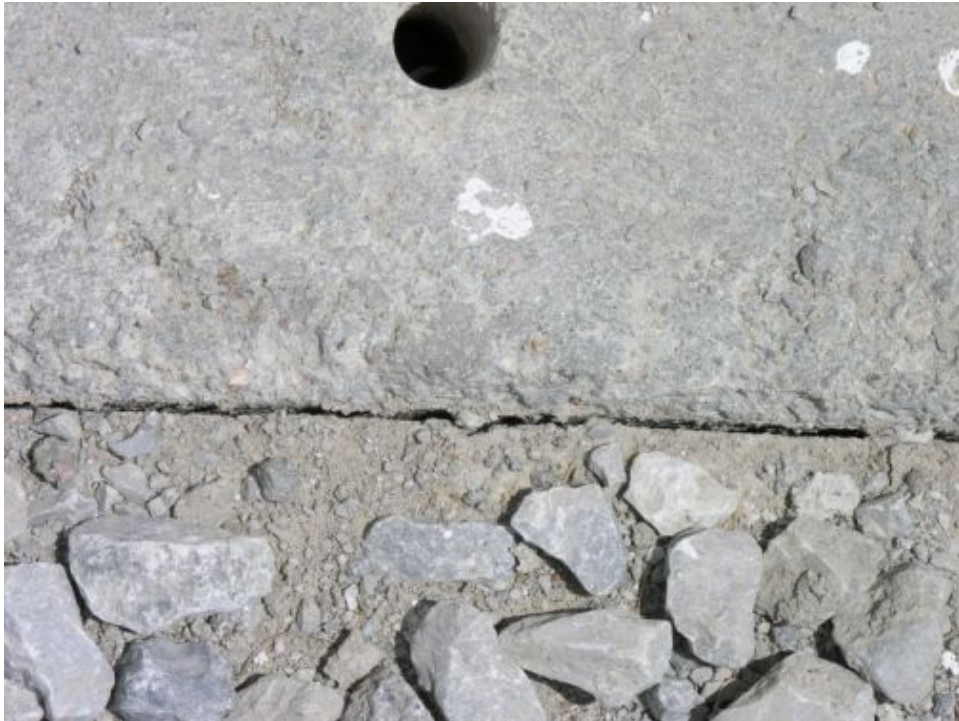
Figure 22. System Damage, Soil Gap, Test CBPP-1
