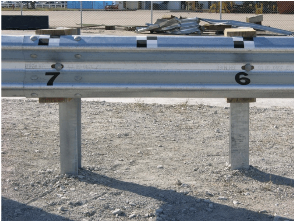
Figure 108. Post Nos. 5 through 7 Damage, Test MWT-5
