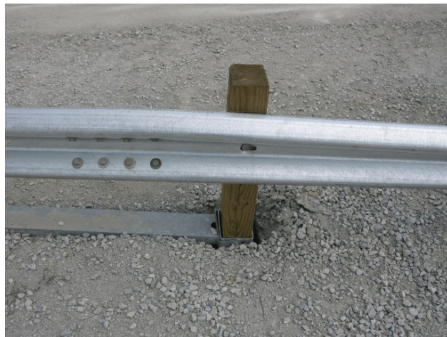
Figure 40. Upstream Anchorage Damage, Test No. MGS221-1
