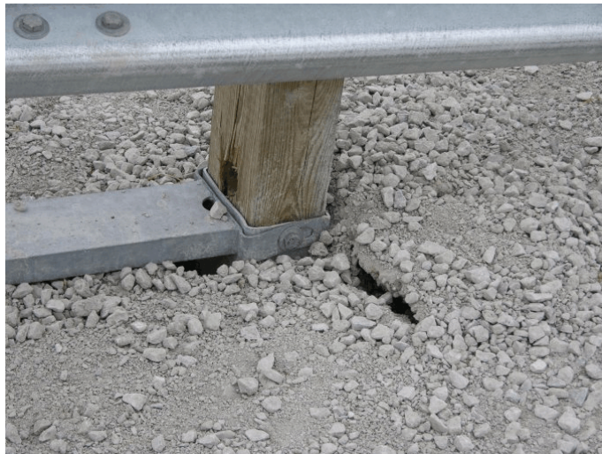
Figure 63. Upstream Anchorage Damage, Test No. MGS221-2
