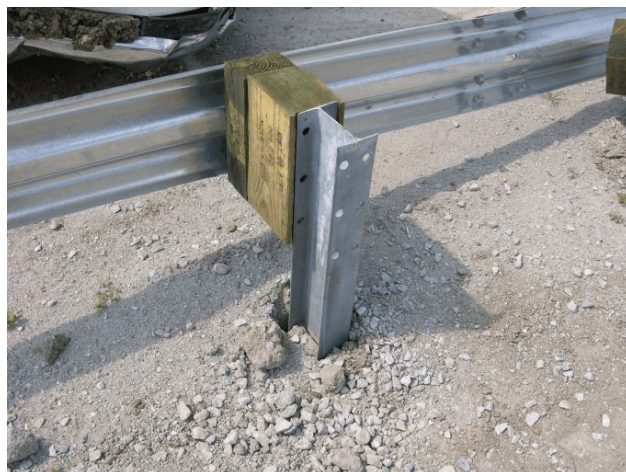
Figure 39. Post Nos. 25 through 27 Damage, Test No. MGS221-1
