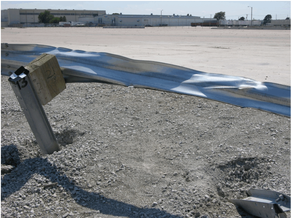
Figure 28. System Damage, Test No. MGSAS-1
