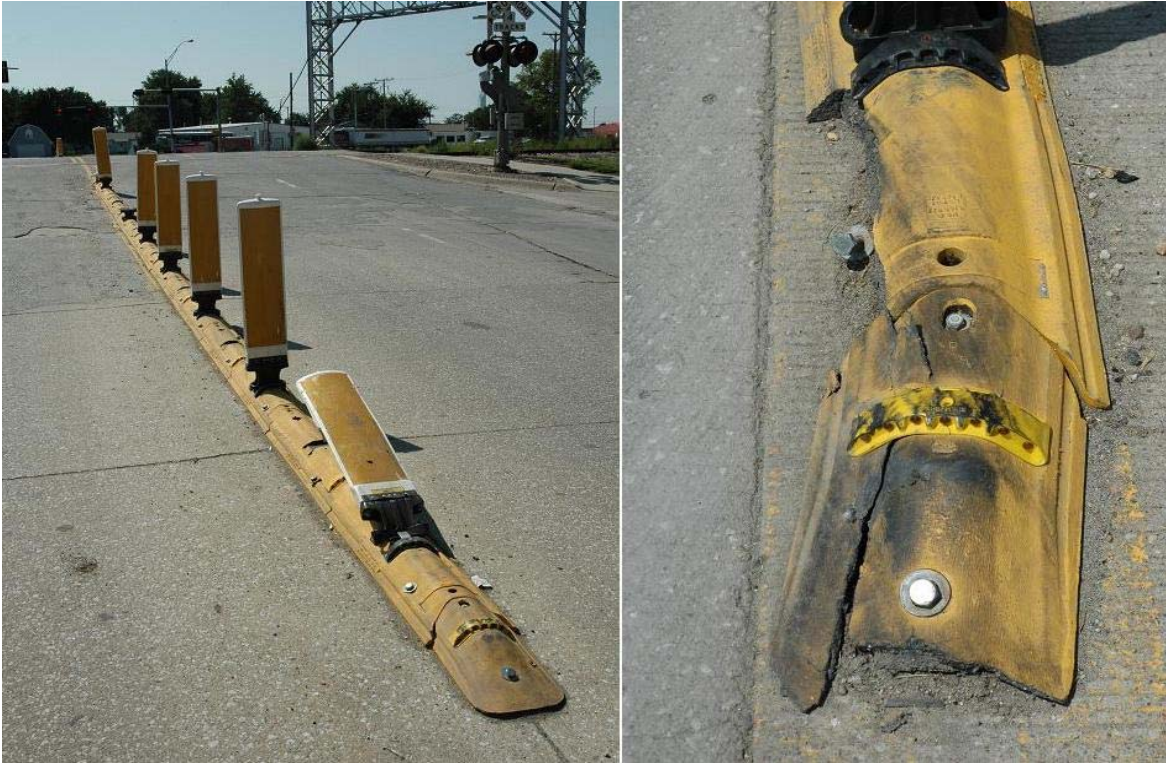
Figure 4.1. Flattened and abused curbing due to overrunning trucks in Waverly
