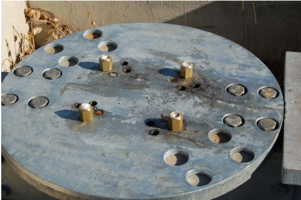
Figure 28. System Damage, Test No. BBC-1
