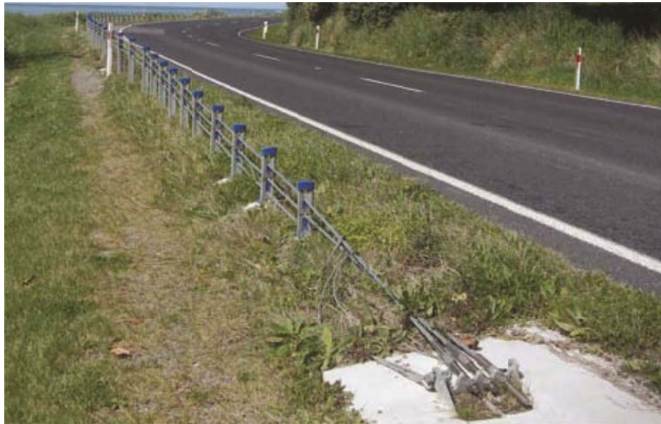
Figure 7. Safence End Terminal
