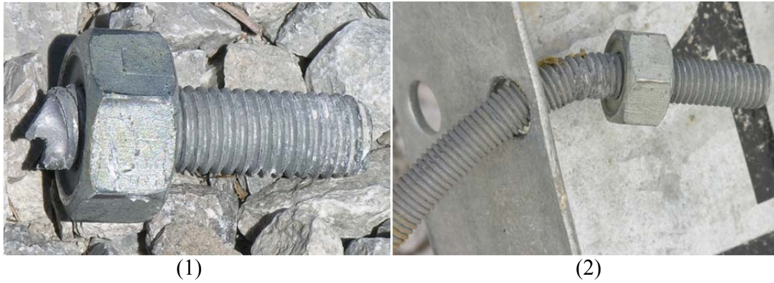
Figure 28. Blockout Bolt Failure Modes
