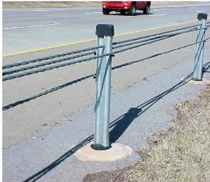
Figure 1.1 Brifen High tension Wire Rope Safety Fence (TL-4)
