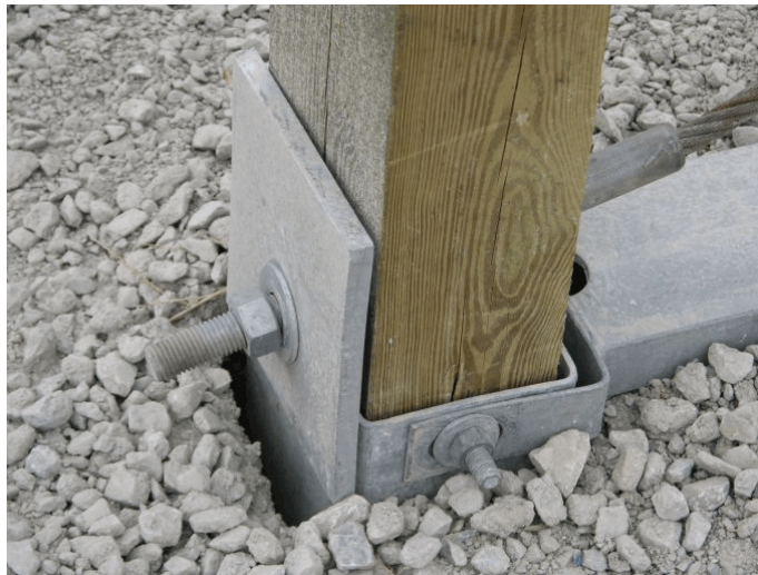
Figure 64. Downstream Anchorage Damage, Test No. MGS221-2
