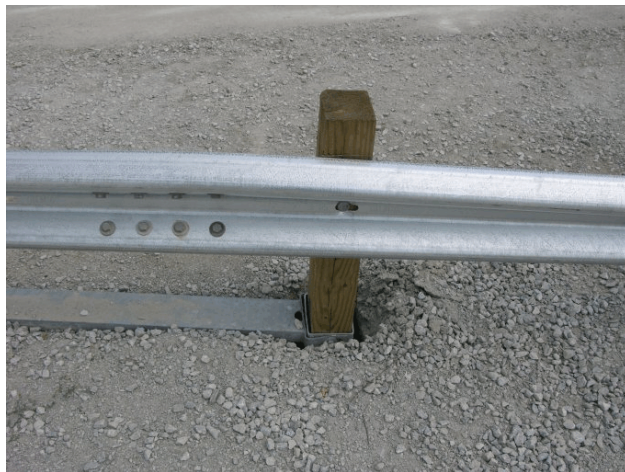
Figure 40. Upstream Anchorage Damage, Test No. MGS221-1
