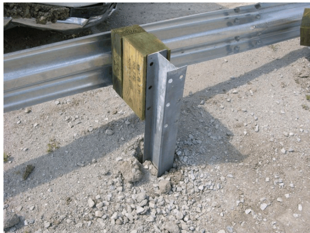
Figure 39. Post Nos. 25 through 27 Damage, Test No. MGS221-1
