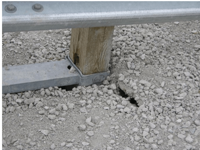
Figure 63. Upstream Anchorage Damage, Test No. MGS221-2
