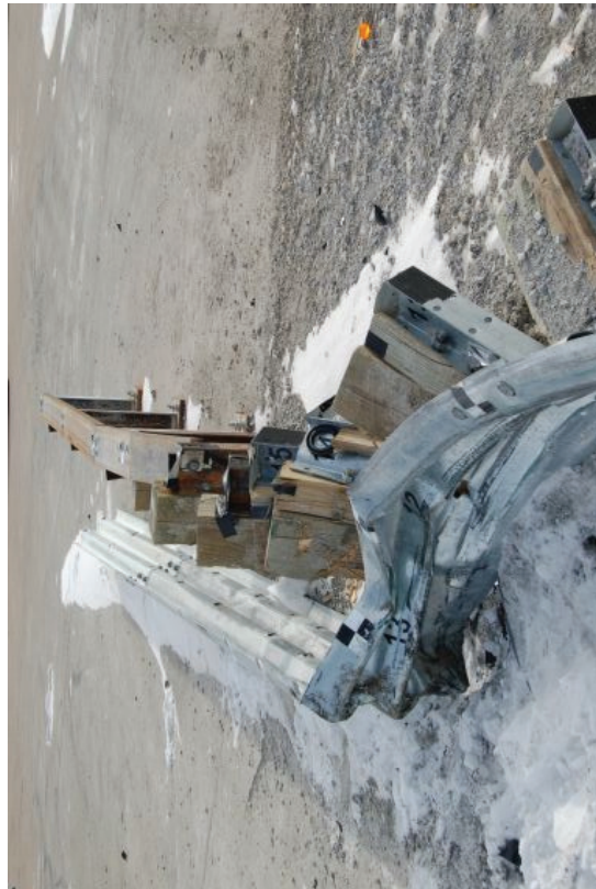
Figure 59. Posts Nos. 13 through 16 Damage, Test No. MWTSP-1
