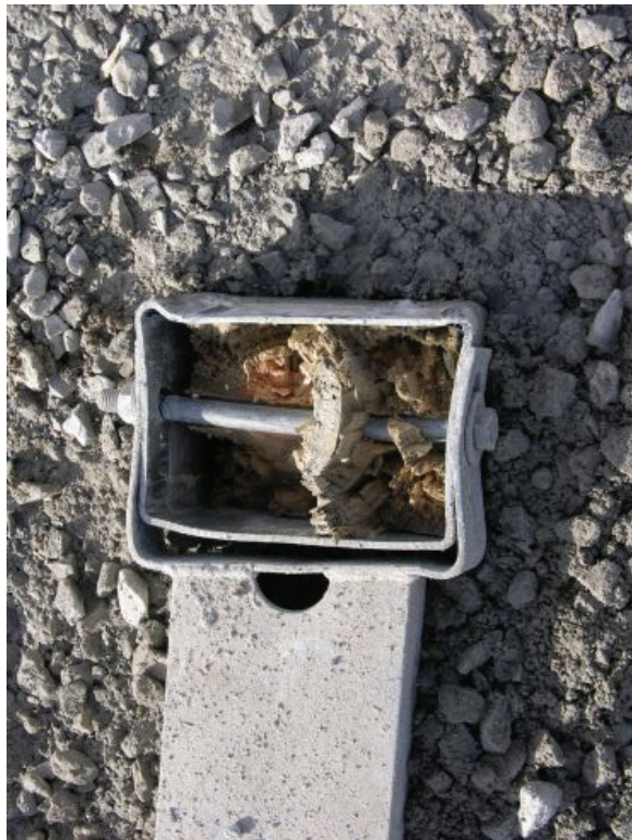
Figure 60. Upstream Anchorage Damage, Test No. MWTSP-1
