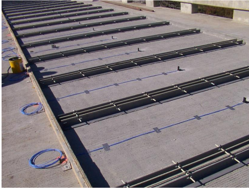
Figure 8. Angle iron electrodes and thermocouple wiring layout
