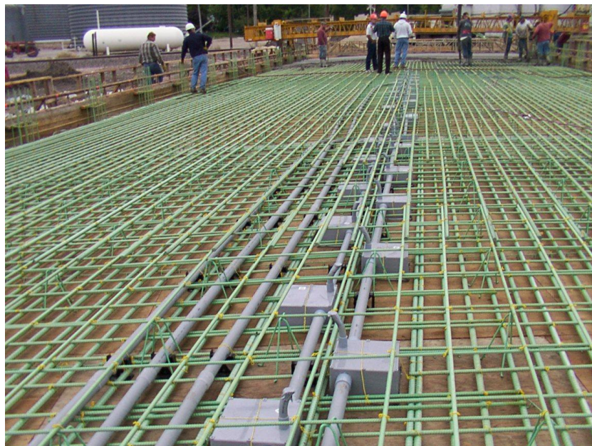
Figure 9. PVC Conduits and Junction Boxes pre-positioned in the Regular Reinforced Concrete Bridge Deck
