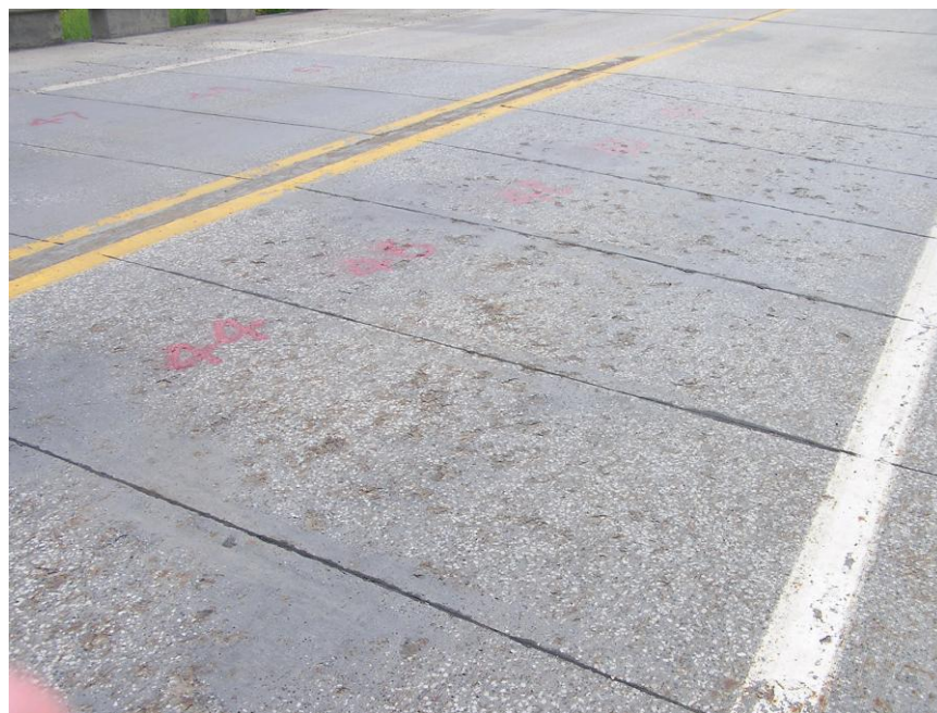
Figure 24. Deterioration of Eastbound Lane Slabs
