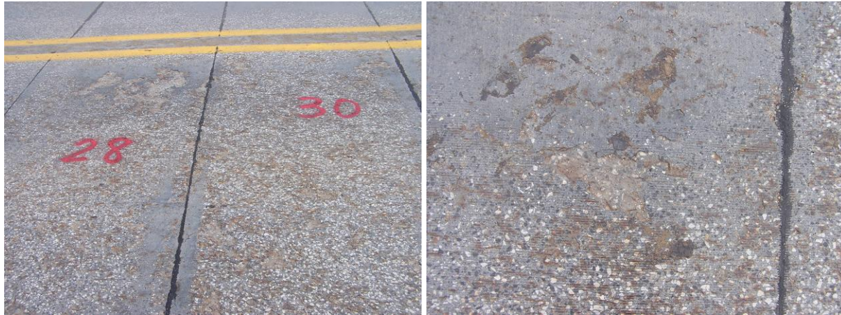
Figure 25. Close-up of Surface Spalls in Eastbound Lane
