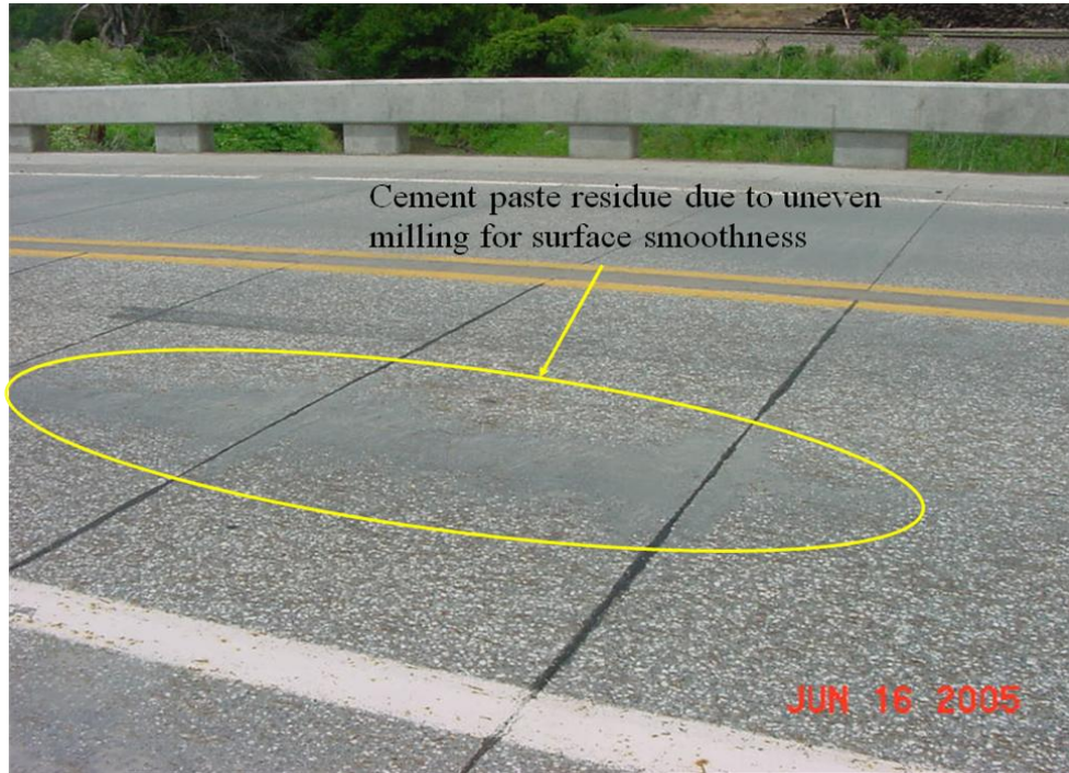
Figure 19. Cement paste cover was milled off leaving steel fibers exposed
