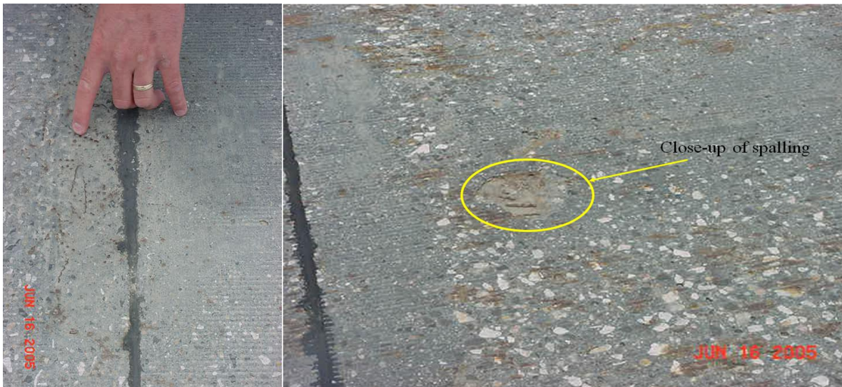
Figure 20. Close-up of exposed steel fibers and spalls
