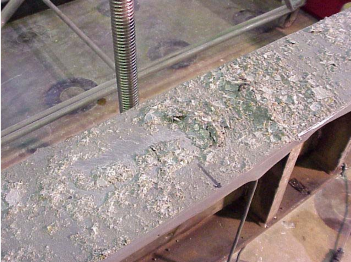
Figure 3-75: Failure Surface Near Mid-Span
