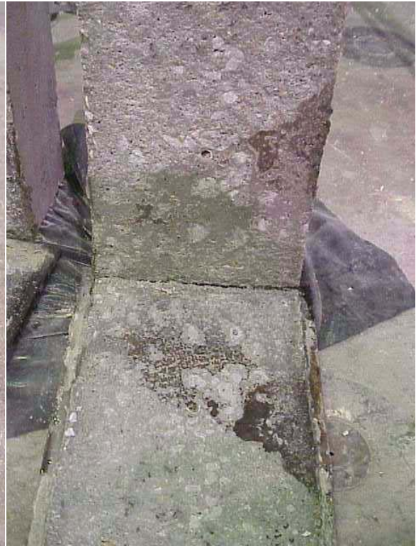
Figure 3-28: Close-up of interface
