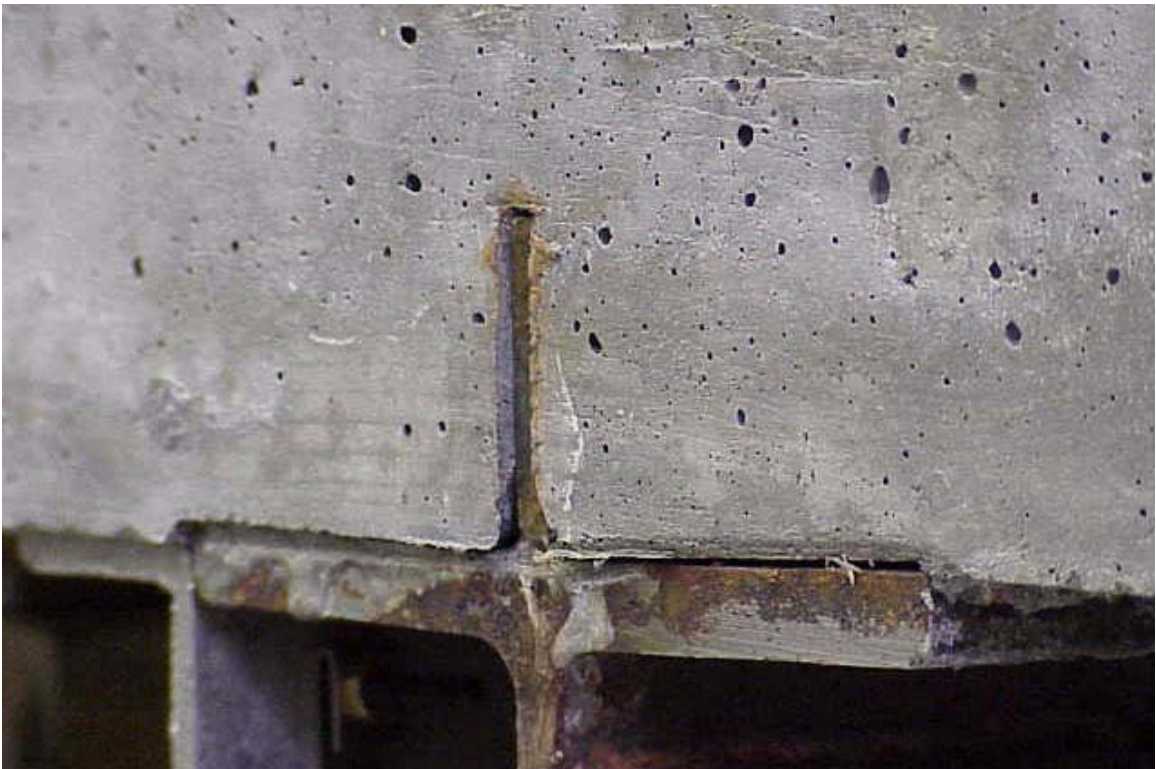
Figure 3-118: Relative Slip of Concrete and Steel at End of Girder
