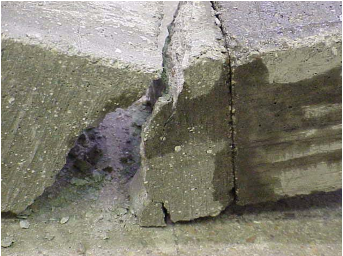
Figure 3-34: Close-up of failure
