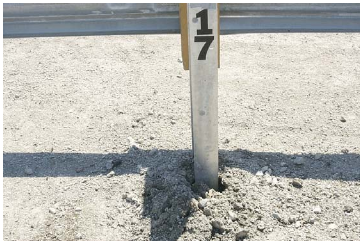
Figure 45. Post Nos. 13, 14, and 17 Damage, Test NPG-1
