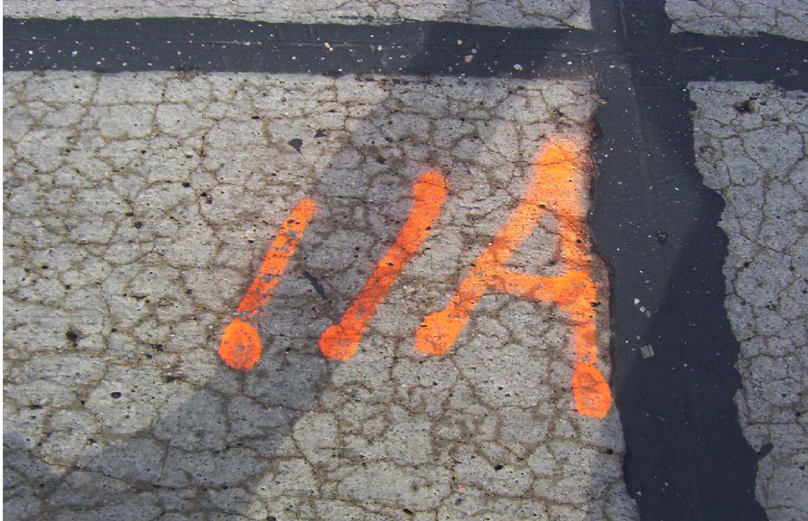
Photo No. 1 - ASR Damage
