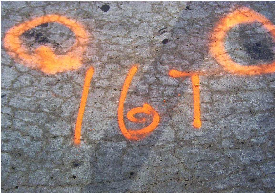
Photo No. 2 - ASR Damage
