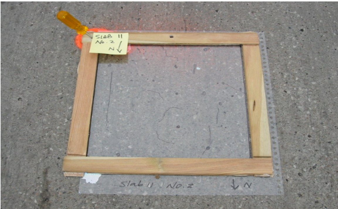
Photo No. 22 – Crack Mapping
