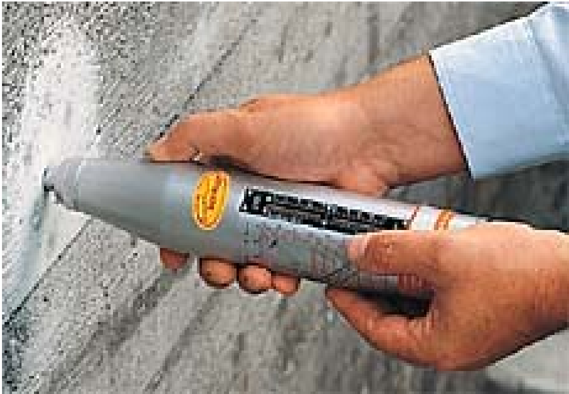
Photo No. 20 – Schmidt Hammer Evaluation
