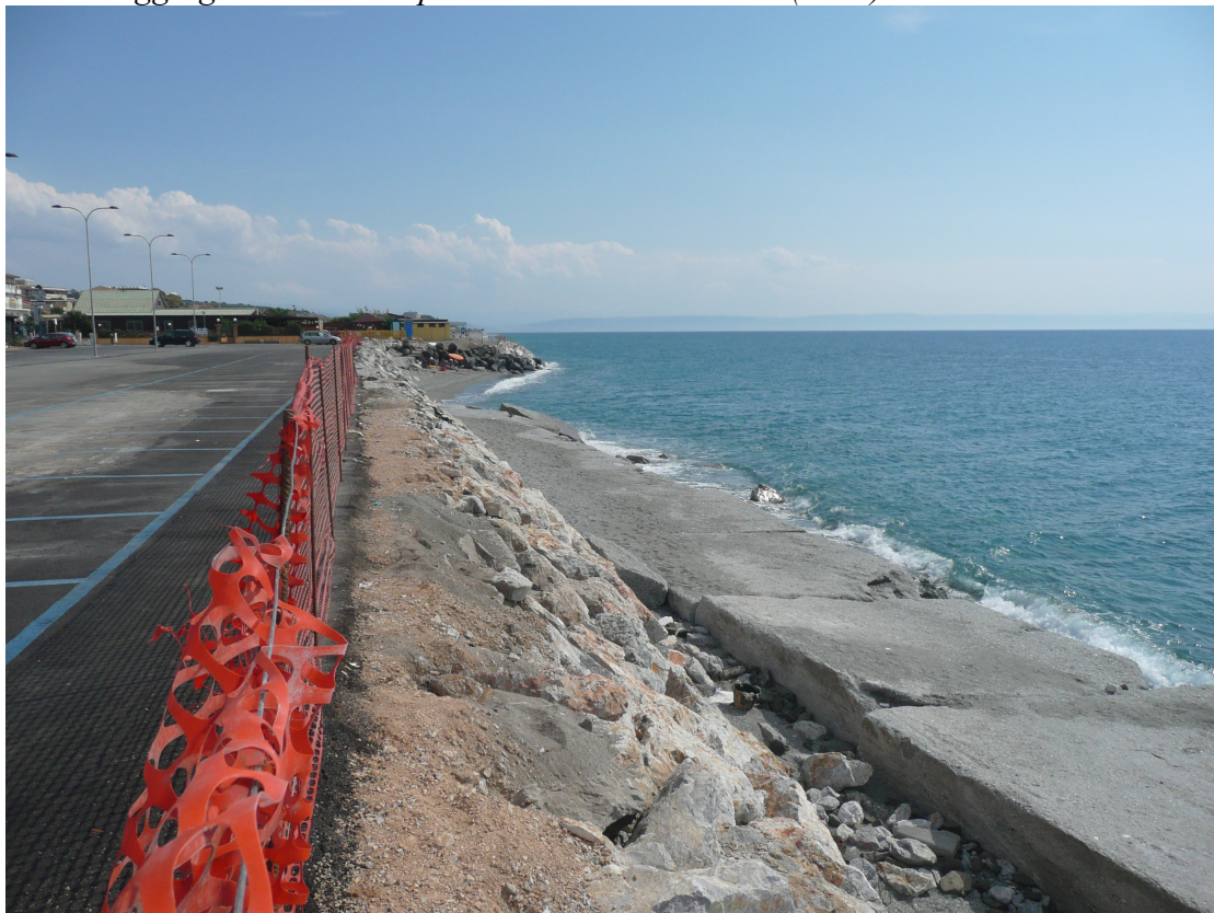
Plate 2 Erosion and coastal defences south of the Fiume Savuto (2009)
