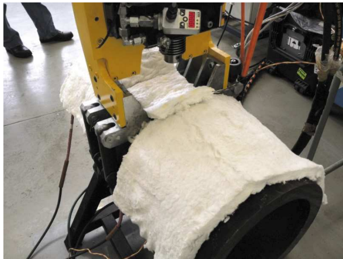
Figure 6. FTHP processing platform in-situ on a section of thick walled steam pipe. The pads are for preheating the pipe to approximately 200°C prior to commencing the WeldCore® process.
