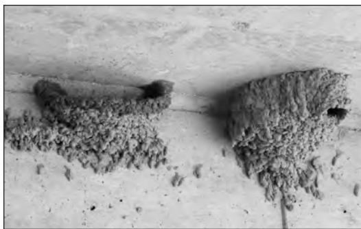
Figure 1. Partial (left) and completed cliff swallow nests on the underside of a bridge.
