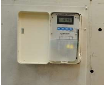
Fig. F.2.2. 120 V timeclock used to control chambers.
