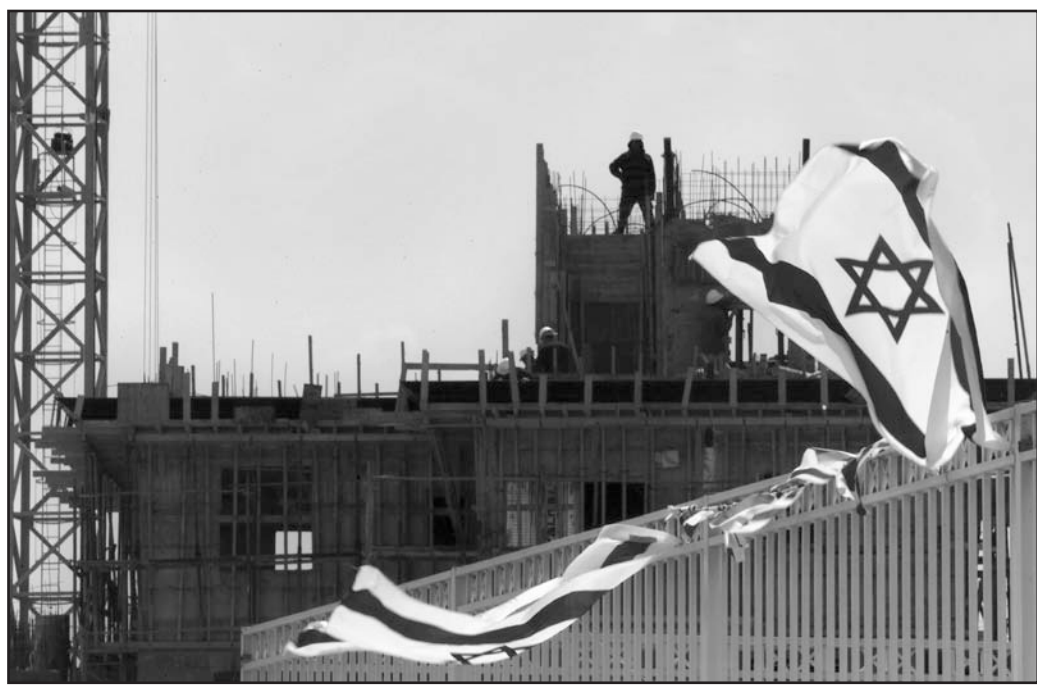
CONSTRUCTION WORKERS work on a new housing development, as an Israeli flag flies in the foreground, in the Jewish neighborhood of Har Homa, in east Jerusalem, Thursday, April 22. Aides to Israel's prime minister said Thursday that he has officially rejected President Barack Obama's demand to suspend all construction in contested east Jerusalem. AP photo
