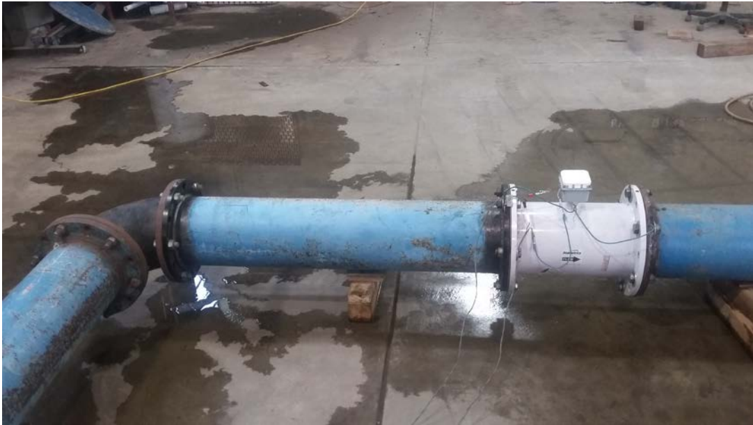
Figure 9. Phase II Elbow Setup for 5D Test (flow left to right)
