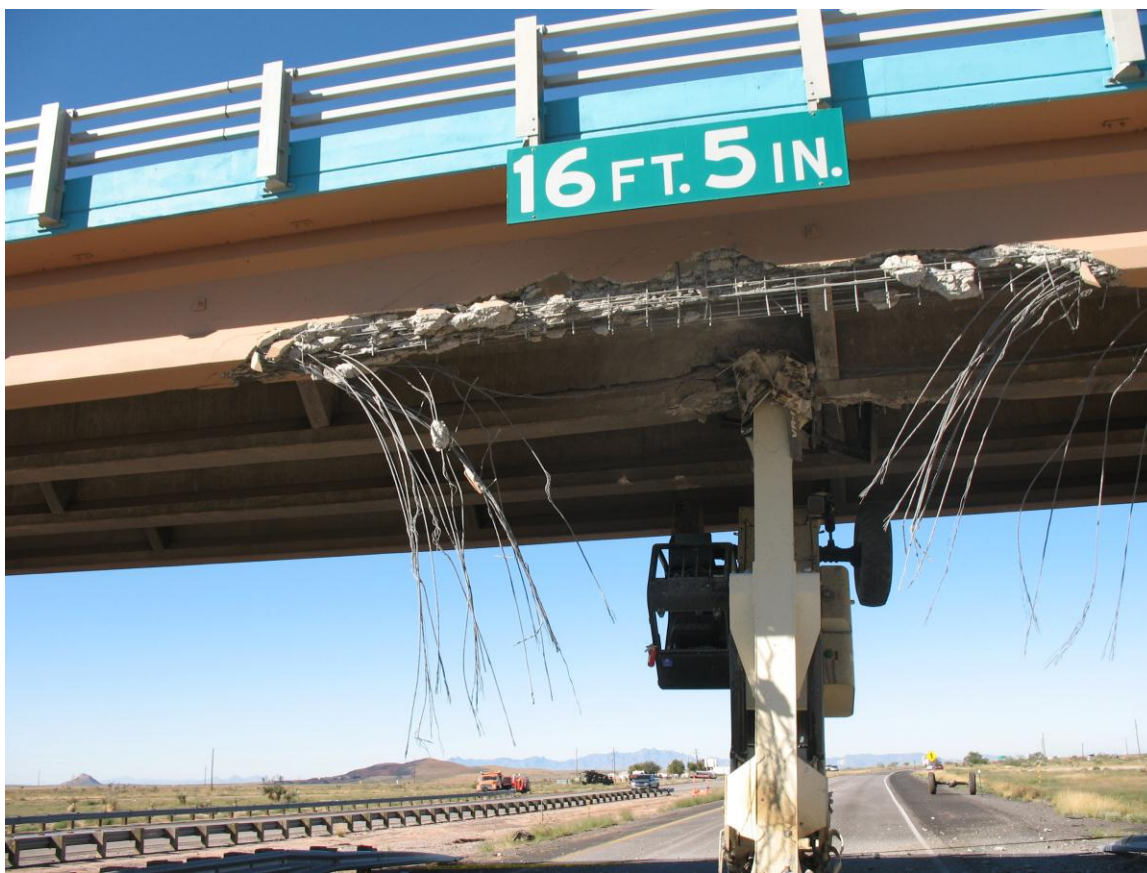
Figure 2 Partial collapse of I-10 underpass in Southern New Mexico.
