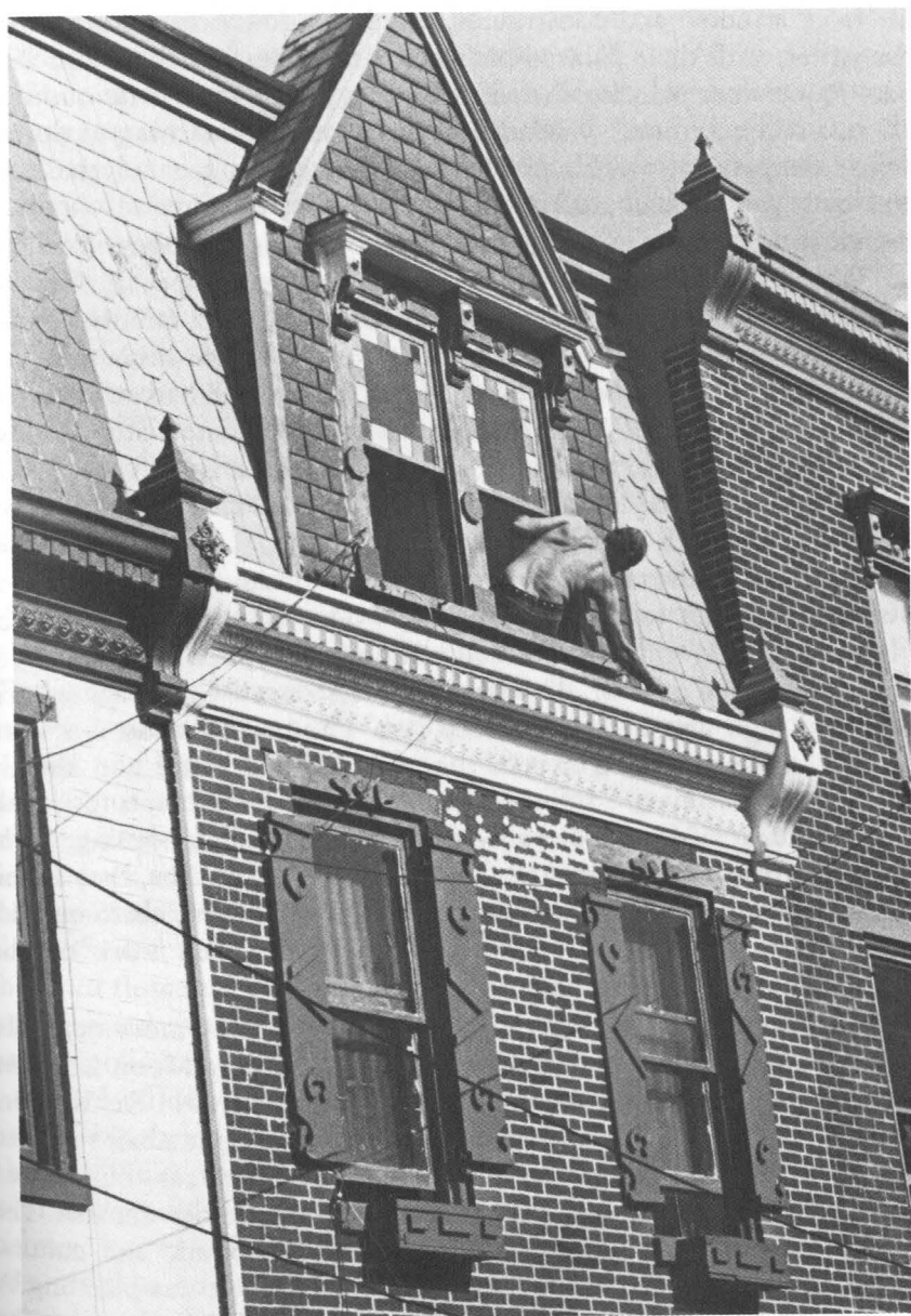
Figure 5-2. Cal Painting over the Facade, after Completing Construction of Shutters from Materials of Other Houses, July 1983 ( Courtesy Simon Bronner )
