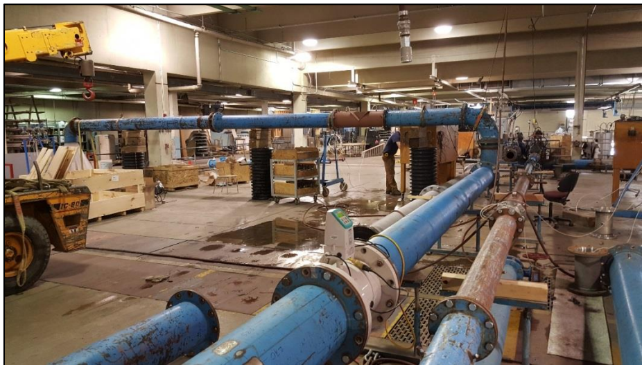
Figure 3: Laboratory Flowmeter Installation
