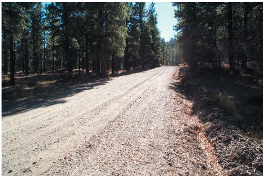
This forest road is located well away from water. Its gravel surface promotes drainage and lessens erosion. The road is crowned, so water drains away to both sides.
