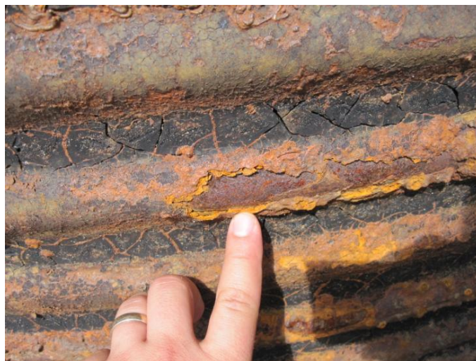
Figure 2. Half-pipe riser weir's sheet metal skin experiencing pitting corrosion after one use cycle with protective asphaltic coating.
