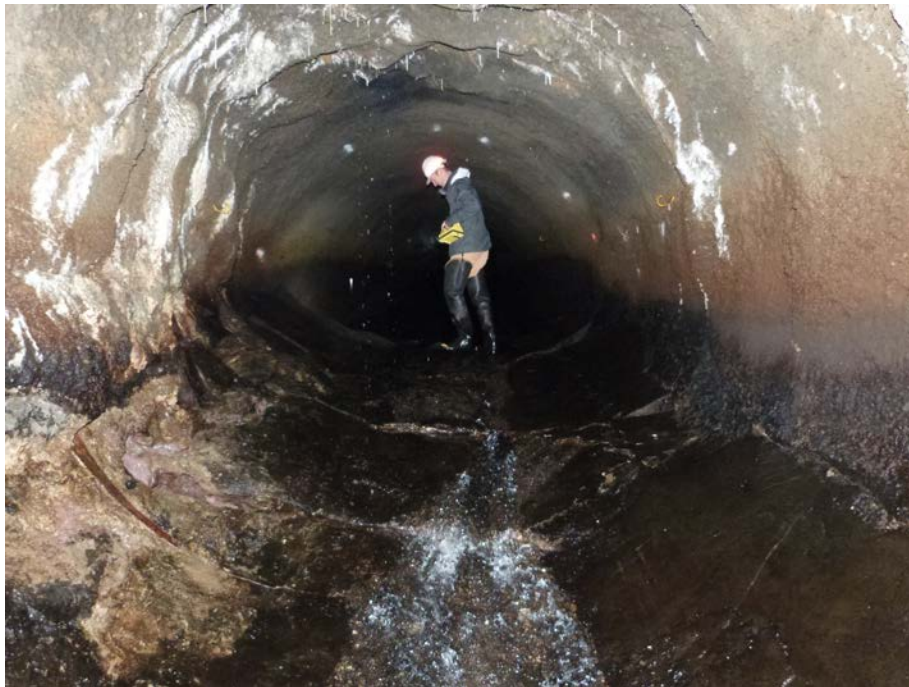
Figure 4. Photo of heave in tunnel
