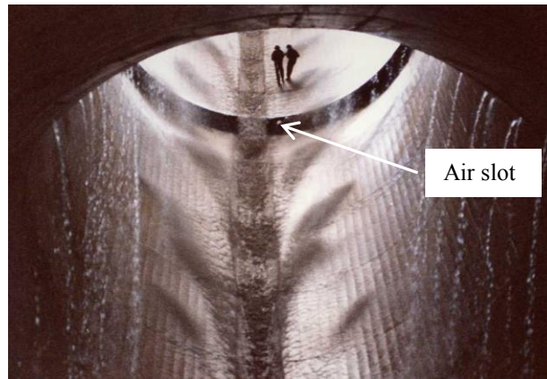
Figure 5. Air Slot at Glen Canyon Dam
