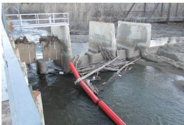
Figure 4. St. Mary Diversion sluiceway gates (view is from upstream left bank, standing on top of the headworks structure)
