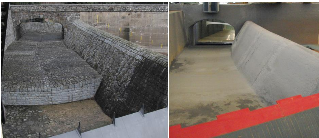
Figure 3. Spillway of the Malter Dam 2014 (left) (Source: LTV); Evened bottom slope in the hydraulic model (right)
