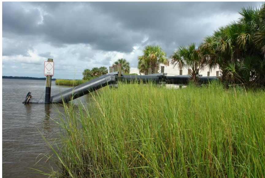
Figure 6. Permanently installed and elevated 30 inch outfall pipes to minimize wetland impacts Bartram Island Cell B2 (Maglio et al. 2014).
