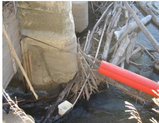
Figure 9. Concrete degradation upstream end of piers surrounding sluiceway bays.
