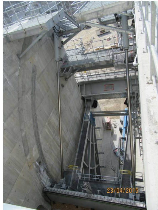
Figure 2. Auxiliary Spillway tainter gate
