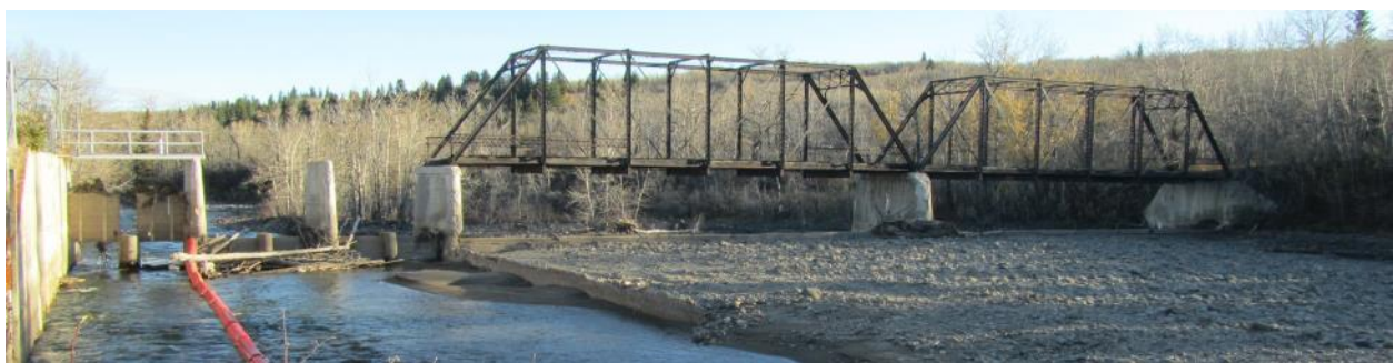
Figure 3. Existing St. Mary Dam Diversion weir, sluiceway and abandoned bridge during low flow fall season (view is from upstream left bank)
