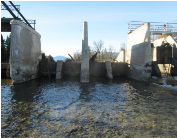
Figure 8. Concrete degradation on the downstream end of piers surrounding sluiceway bays.
