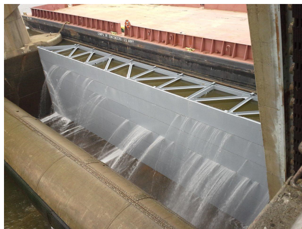
Figure 13. Stoplogs at Winfield Locks and Dam, USA (USACE Huntington District)
