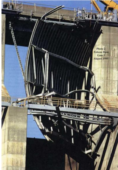
Figure 6 – Failure of Radial Gate No.3 at Folsom Dam
