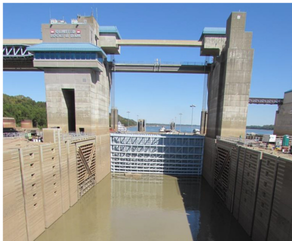
Figure 6. Operational Bulkheads at Olmsted Locks and Dam Project, USA (USACE Louisville District)
