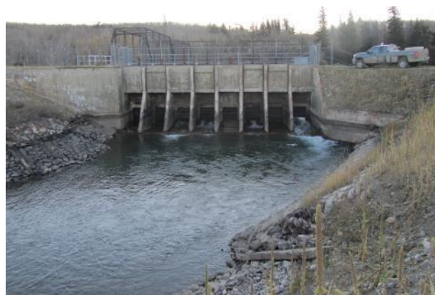
Figure 5. St. Mary Diversion headworks structure (view of from downstream of the headworks, flow is towards reader)
