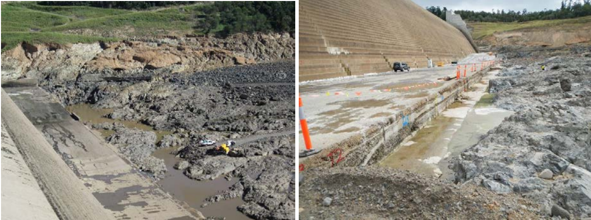
Figure 5. 2013 flood scour downstream of the primary spillway
