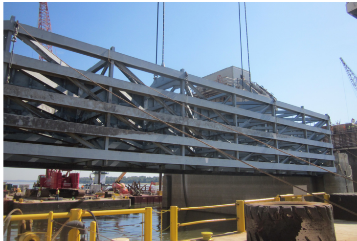
Figure 5. Bulkhead Installation at Olmsted Locks and Dam Project, USA (USACE Louisville District)
