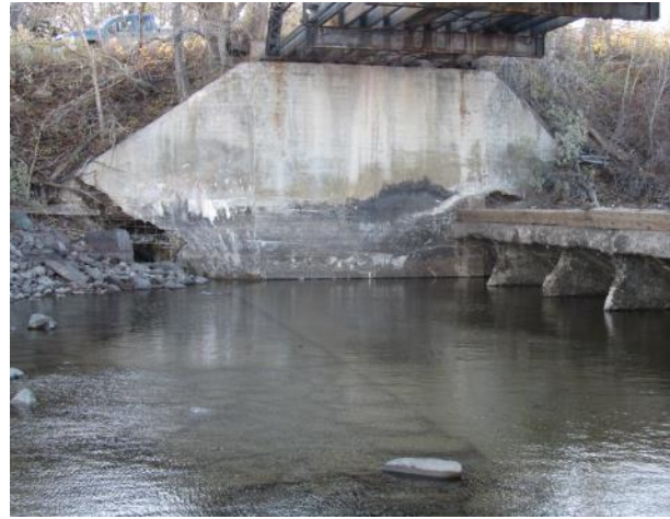
Figure 7. St. Mary Diversion right abutment damage and exposed rebar.
