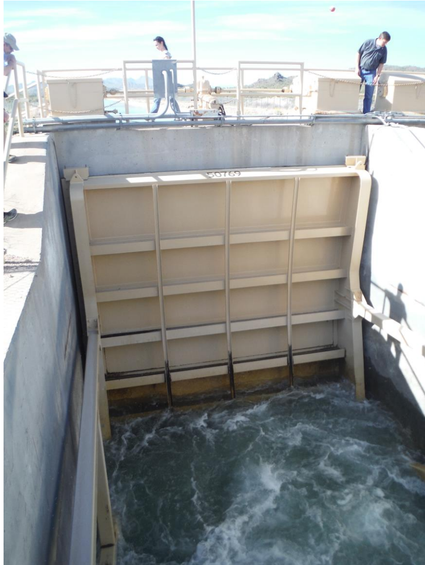
Figure 6. Typical radial gate at a check structure on the CAP Canal
