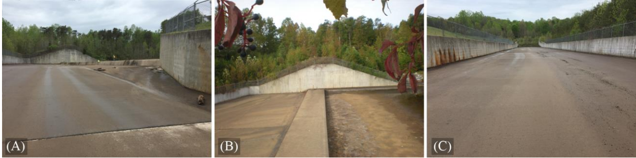
Figure 1. The Existing Auxiliary Spillway for West Fork of Eno River Reservoir Dam looking upstream at control section (A), control section (B), and chute (C)
