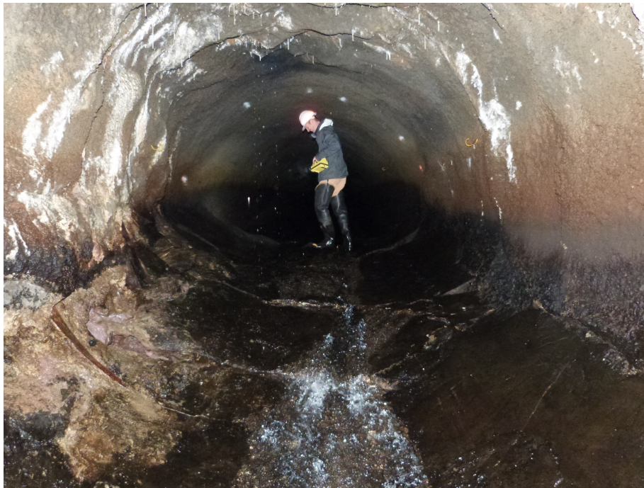
Figure 4. Photo of heave in tunnel
