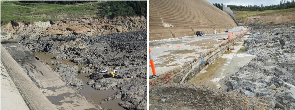
Figure 5. 2013 flood scour downstream of the primary spillway
