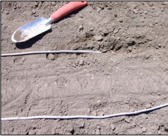
Image 2. Buried electric heating cables.
