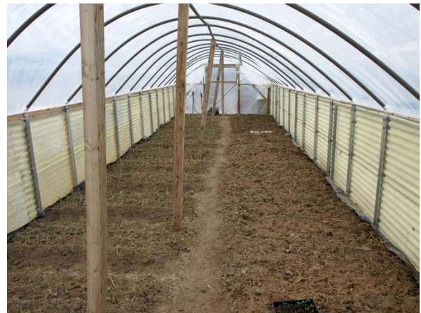
Figure 21. 2x4s can brace the arch during light snow loads. This is a narrower high tunnel but the concept is the same.
