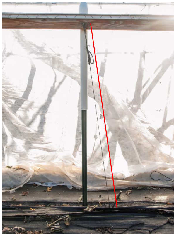
Figure 11. Ground anchor offset slightly and angled into the ground. The white background is actually inside the high tunnel.
