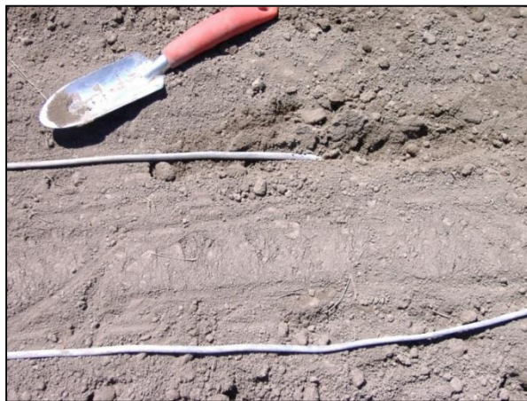
Image 1. Electric heating cable partially buried in soil.
