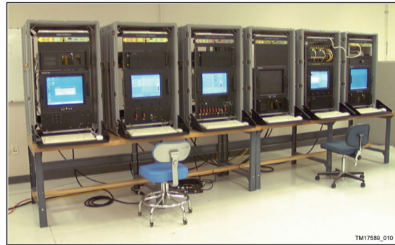
Figure 12 - OSP -Standard Portable Launch Control Consoles
