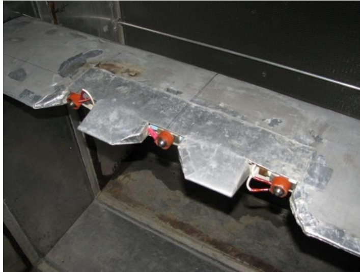
Figure A-2: CAIRWT's Spray Bars with Heating Element
