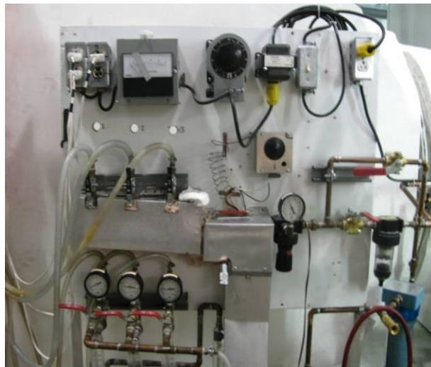
Figure 3-3: CAIRWT's Control Panel
