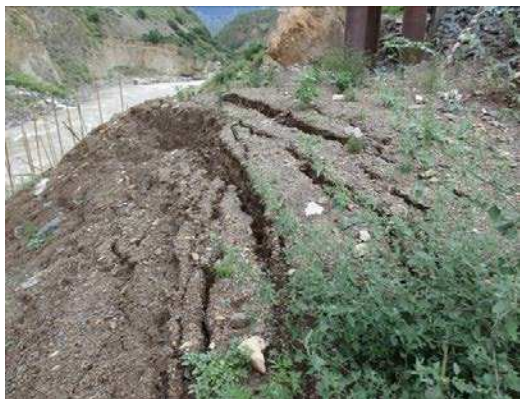
Fig. 17. New emerging arc tensile cracks on the artificial slope (photo taken February 2014)
