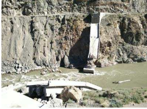
Fig. 18. Dongla Bridge was dismantled by bomb explosion on 12 th July 2015.
